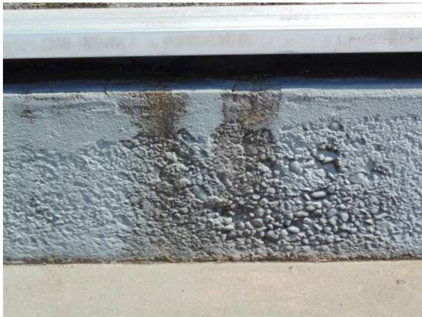
FIGURE B1B: MINOR SPALLING IN CONCRETE
