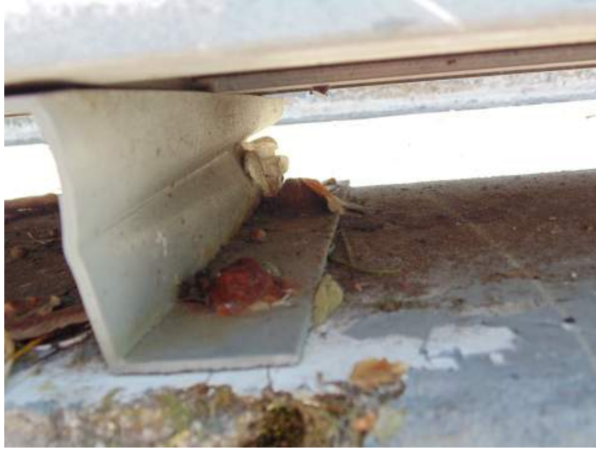
FIGURE B3: RUSTED ANCHOR BOLTS
