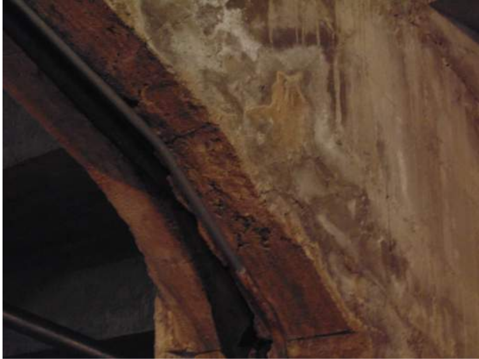
FIGURE C1D-2: CRACKING/SPALLING IN CONC. GIRDER
