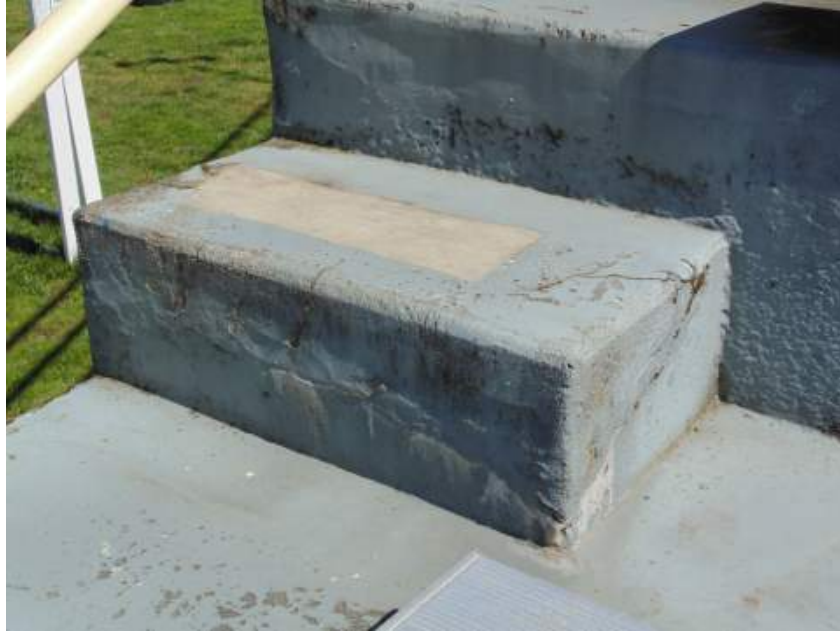
FIGURE B2A: MAJOR CRACKING IN CONCRETE
