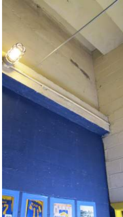
FIGURE C3D-2: CRACK IN CONC. WALL
