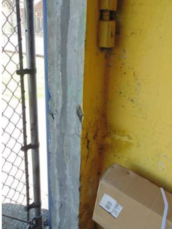
FIGURE C2B-1: CRACKING/SPALLING IN CONC. COLUMN
