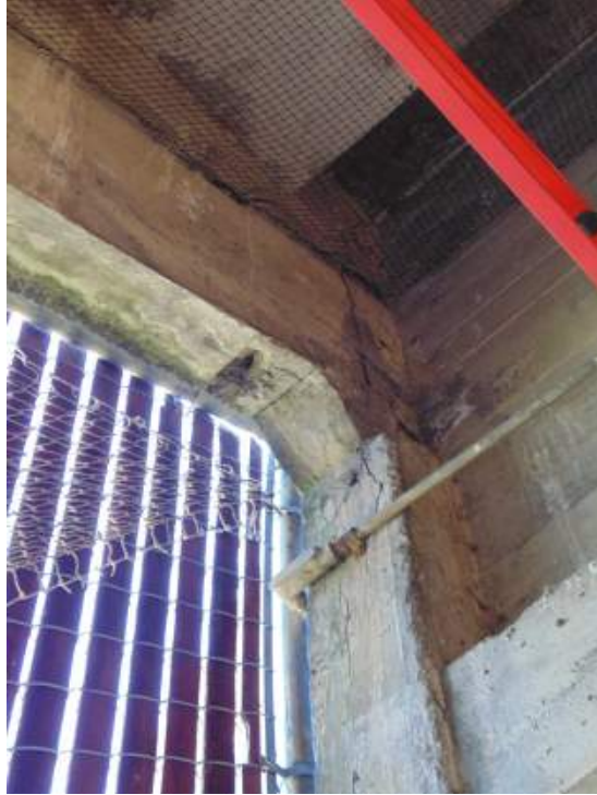
FIGURE C1A-7: CRACKING/SPALLING IN CONC. GIRDER
