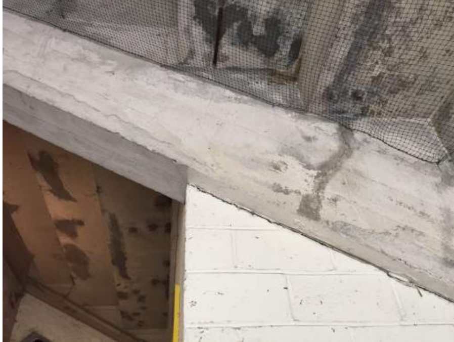
FIGURE C1B-2: CRACKING/SPALLING IN CONC. GIRDER
