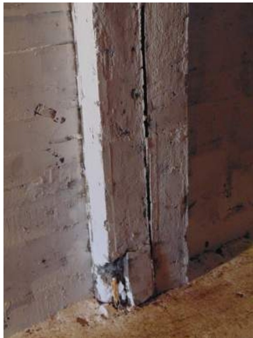
FIGURE C2E: CRACKING/SPALLING IN CONC. COLUMN
