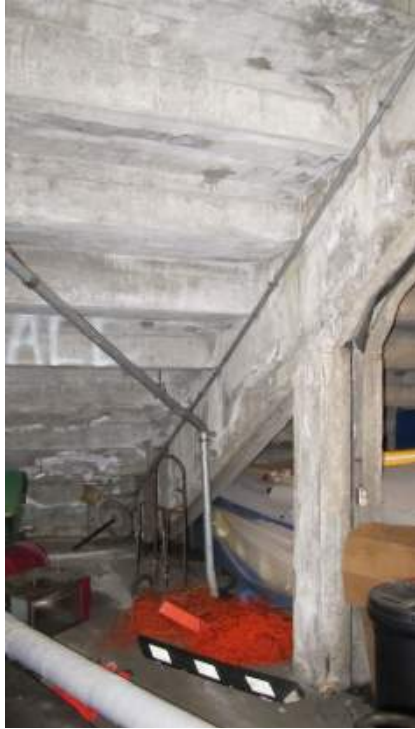
FIGURE C1D-4: CRACKING/SPALLING IN CONC. GIRDER
