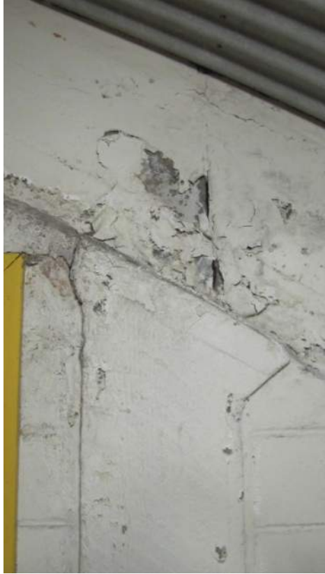
FIGURE C1E: CRACKING/SPALLING IN CONC. GIRDER
