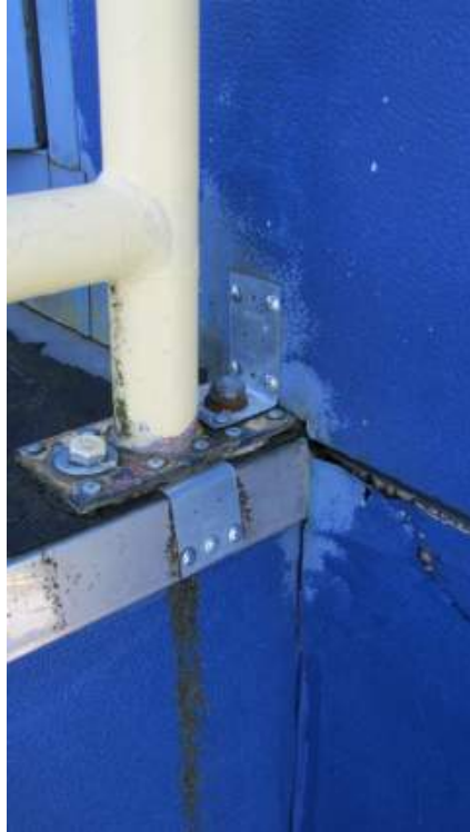
FIGURE B7: RUSTED STEEL CONNECTIONS
