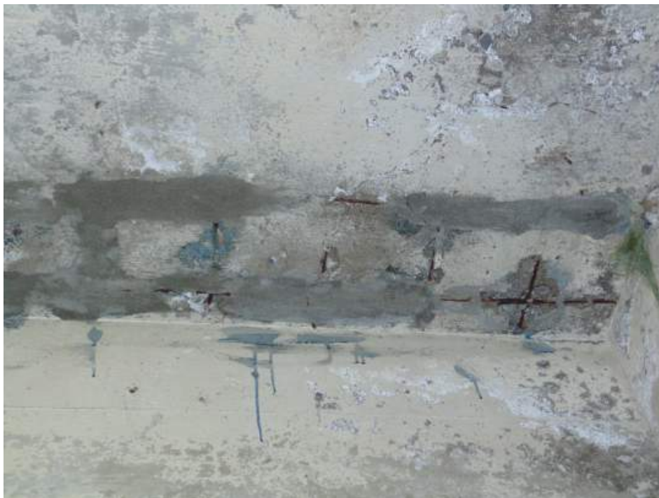
FIGURE C6B: SPALLING/CRACKING/EXPOSED STEEL ON UNDERSIDE OF BEAMS
