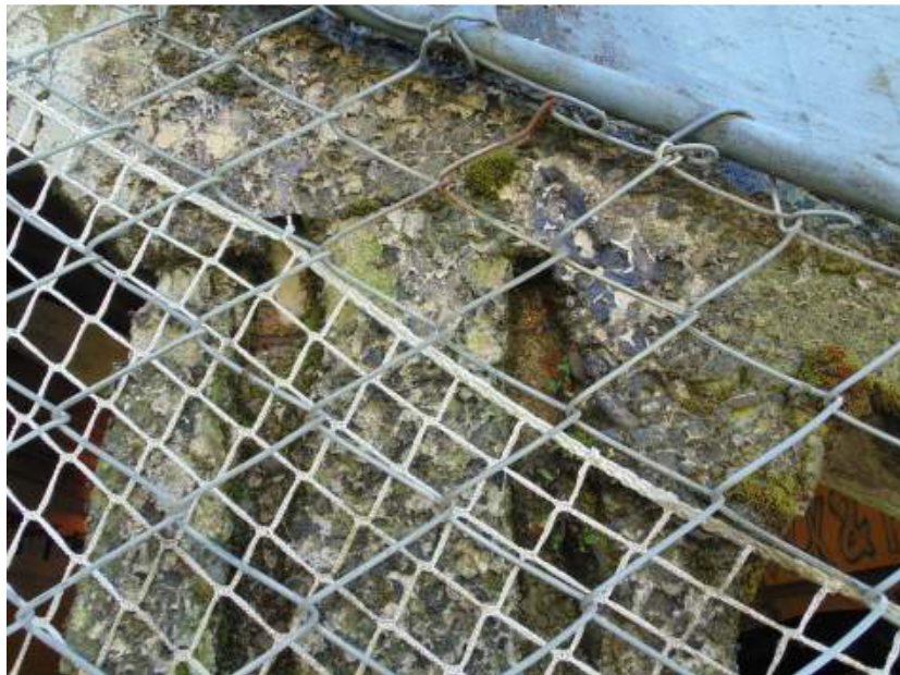
FIGURE C2A: CRACKING/SPALLING IN CONC. COLUMN
