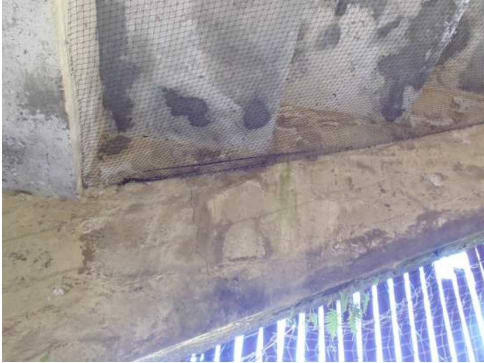
FIGURE C1A-3: CRACKING/SPALLING IN CONC. GIRDER
