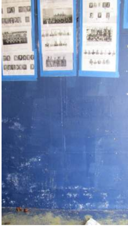
FIGURE C4B: SPALL IN CONC. WALL
