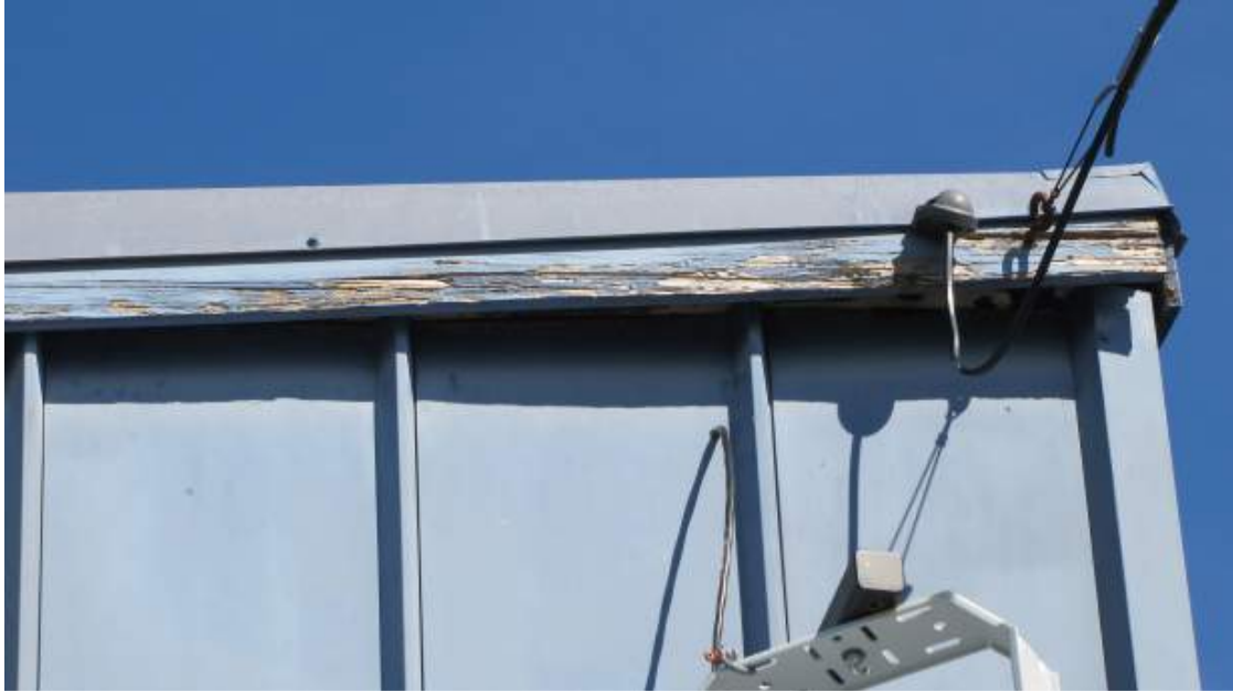
FIGURE W1: WOOD DETERIORATING AT PRESS BOX
