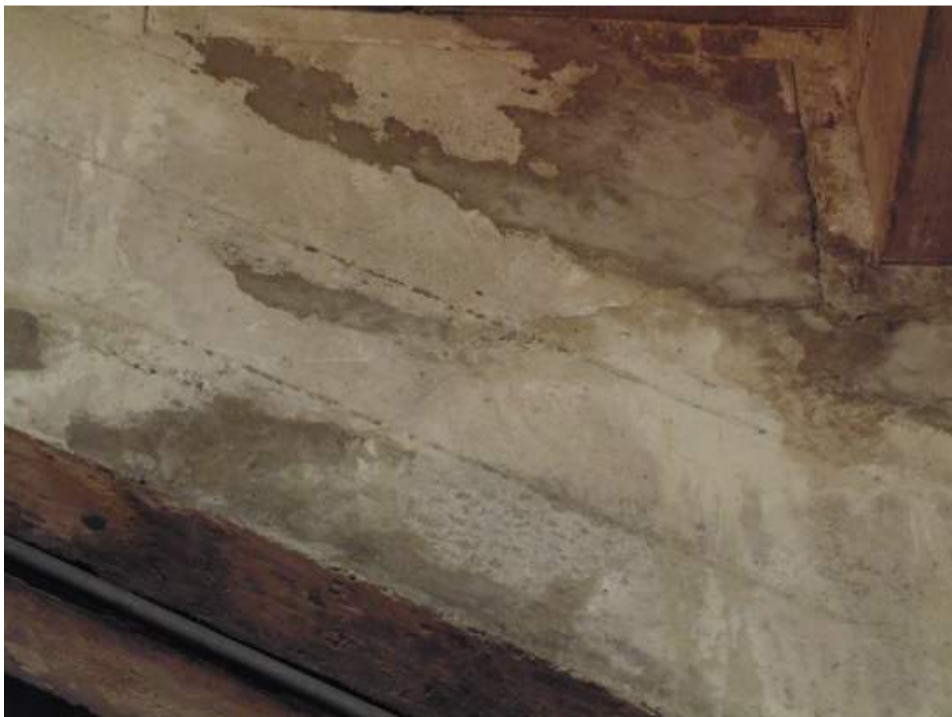
FIGURE C1D-6: CRACKING/SPALLING IN CONC. GIRDER
