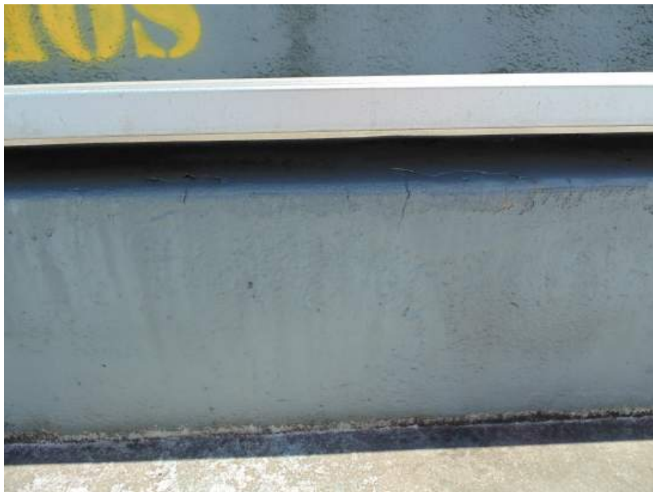
FIGURE B2B: MINOR CRACKING/SURFACE DETERIORATION IN CONCRETE
