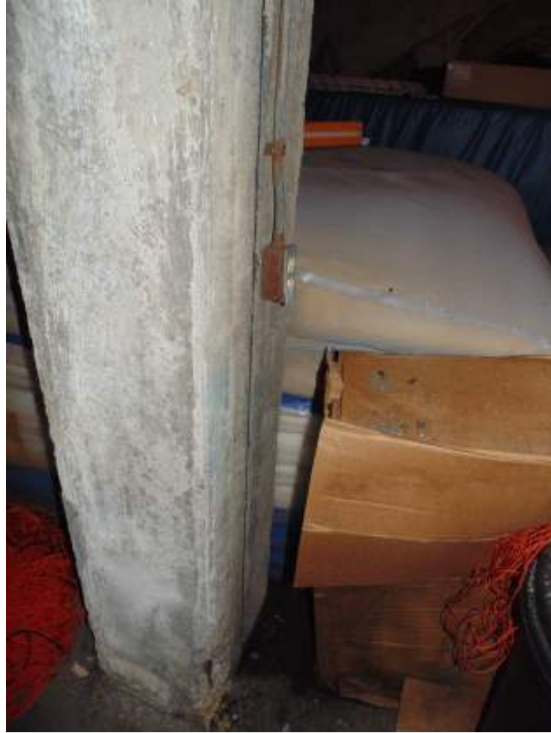
FIGURE C2D: CRACKING/SPALLING IN CONC. COLUMN
