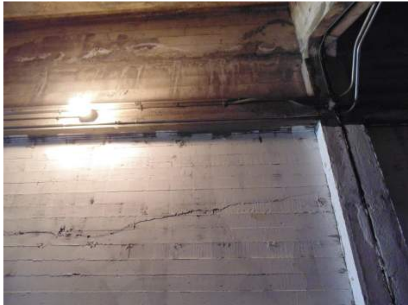
FIGURE C3B: CRACK IN CONC. WALL
