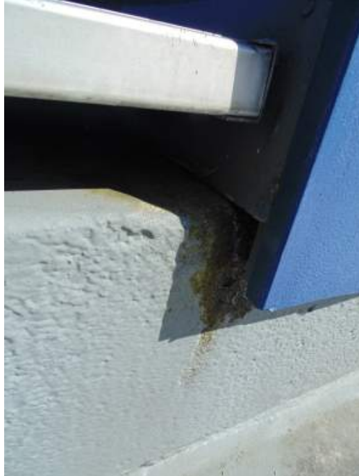
FIGURE B5: RUST AT PRESS BOX
