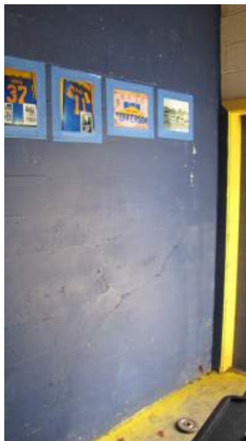
FIGURE C3D-1: CRACK IN CONC. WALL
