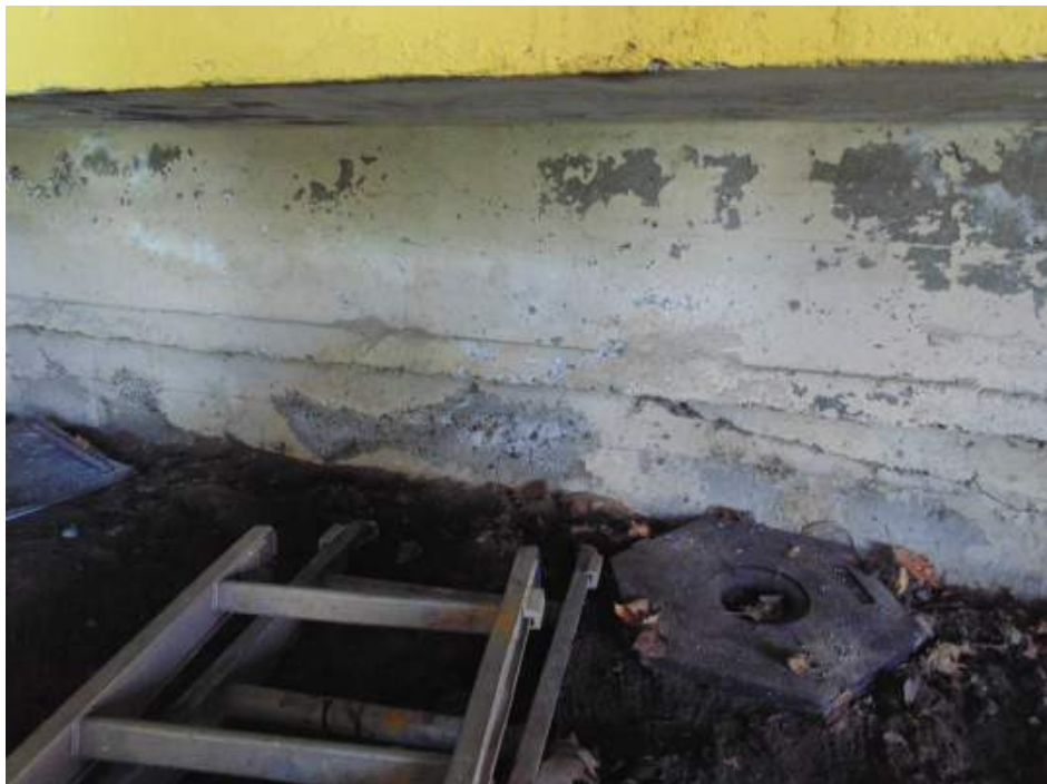
FIGURE C5: SPALLING/CRACKING IN STEM WALL
