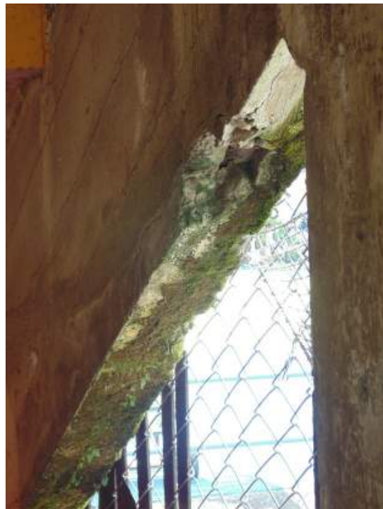
FIGURE C1A-4: CRACKING/SPALLING IN CONC. GIRDER
