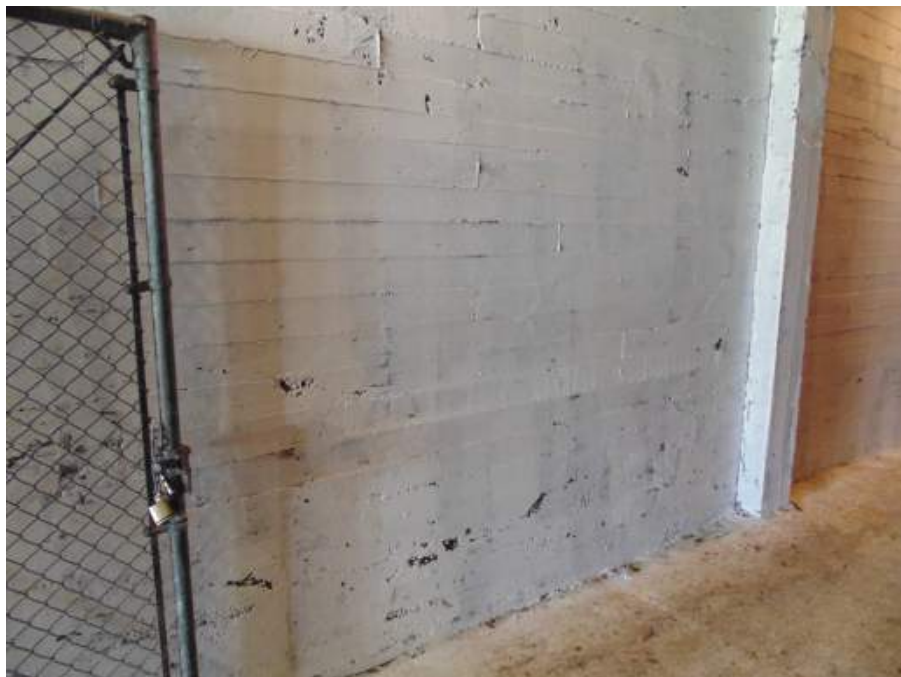
FIGURE C4A: SPALL IN CONC. WALL
