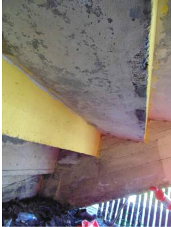
FIGURE C6A: SPALLING/CRACKING/EXPOSED STEEL ON UNDERSIDE OF BEAMS
