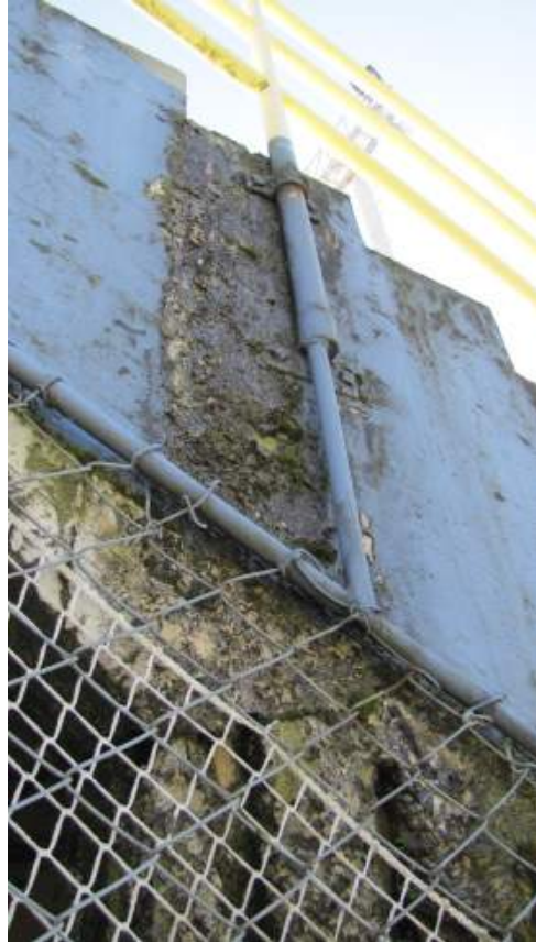
FIGURE C1A-5: CRACKING/SPALLING IN CONC. GIRDER
