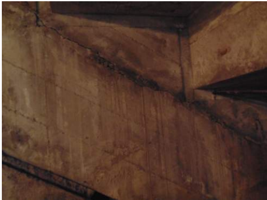
FIGURE C1D-1: CRACKING/SPALLING IN CONC. GIRDER
