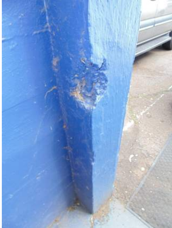
FIGURE C2F-1: CRACKING/SPALLING IN CONC. COLUMN
