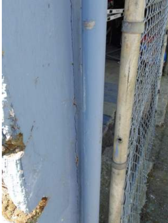
FIGURE C2B-3: CRACKING/SPALLING IN CONC. COLUMN
