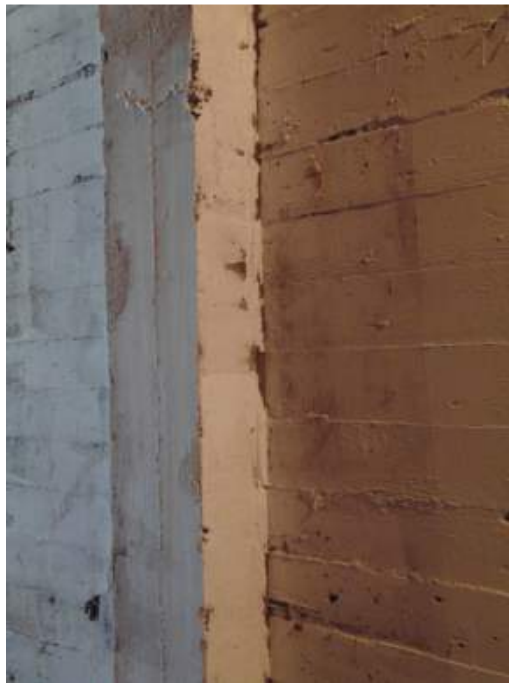
FIGURE C2C: CRACKING/SPALLING IN CONC. COLUMN
