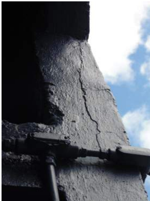
FIGURE C2F-2: CRACKING/SPALLING IN CONC. COLUMN
