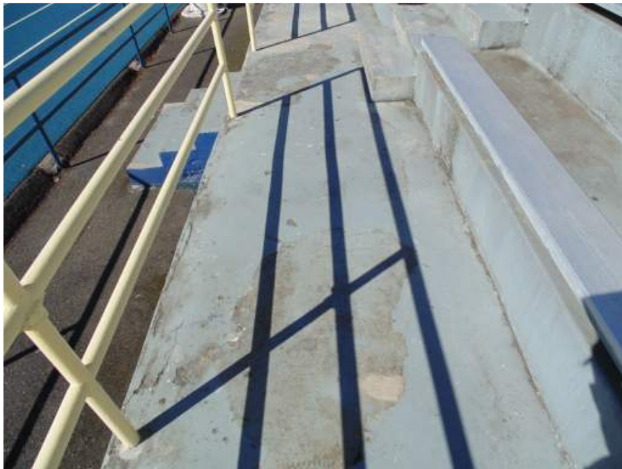
FIGURE B8: DAMAGED/MISSING FINISH
