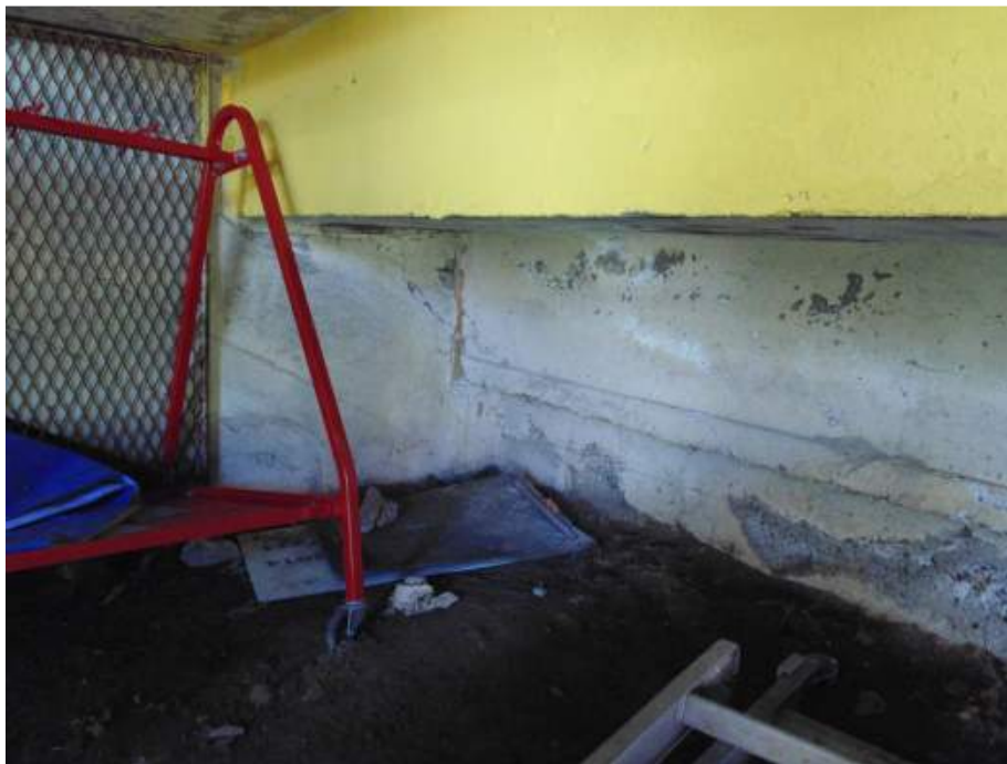
FIGURE C1B-1: CRACKING/SPALLING IN CONC. GIRDER
