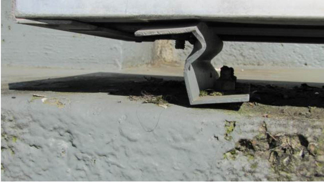
FIGURE B9: DAMAGED SEAT BRACKETS
