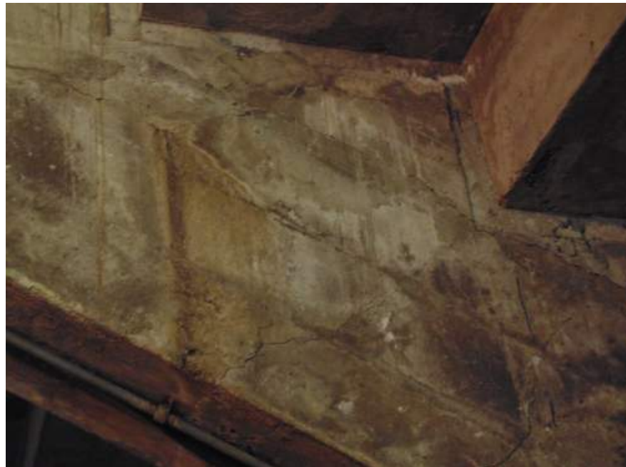
FIGURE C1D-3: CRACKING/SPALLING IN CONC. GIRDER
