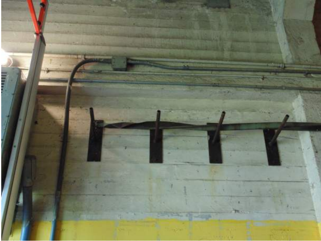
FIGURE C3A: CRACK IN CONC. WALL
