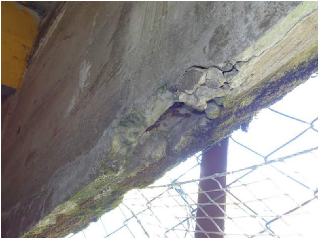
FIGURE C1A-2: CRACKING/SPALLING IN CONC. GIRDER
