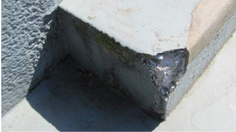
FIGURE B1A: MAJOR SPALLING IN CONCRETE
