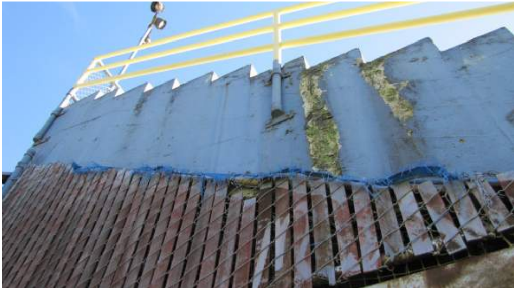
FIGURE C1A-6: CRACKING/SPALLING IN CONC. GIRDER
