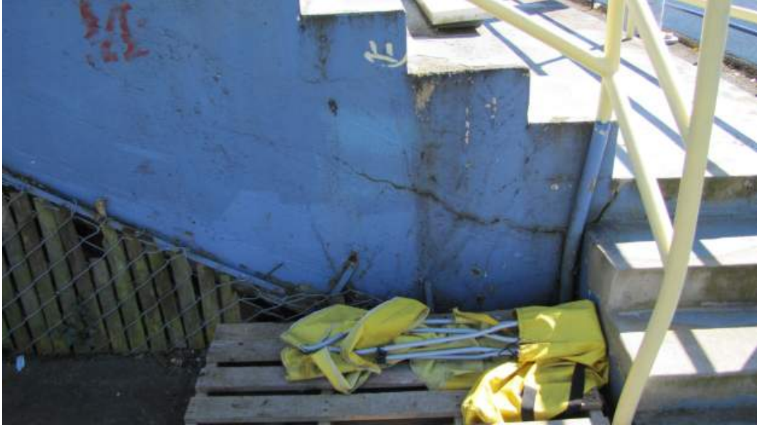
FIGURE C1A-1: CRACKING/SPALLING IN CONC. GIRDER
