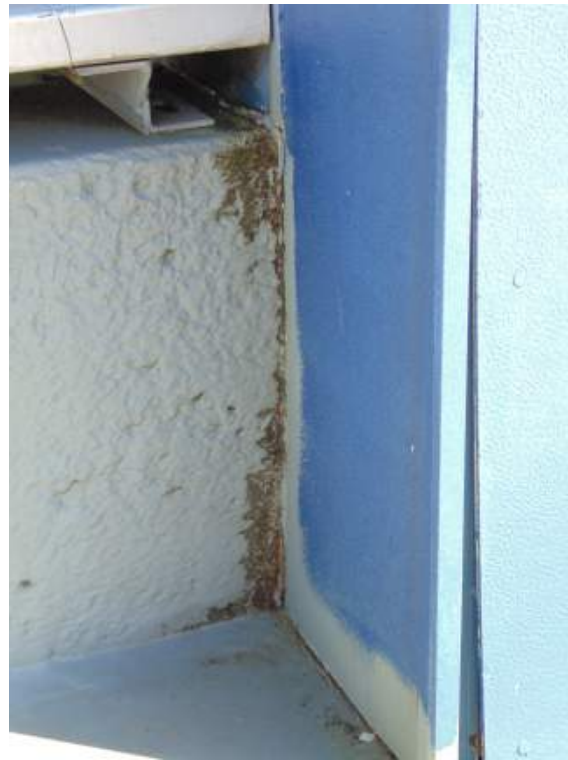
FIGURE B4: MISSING BOLT AT SEAT BRACKET
