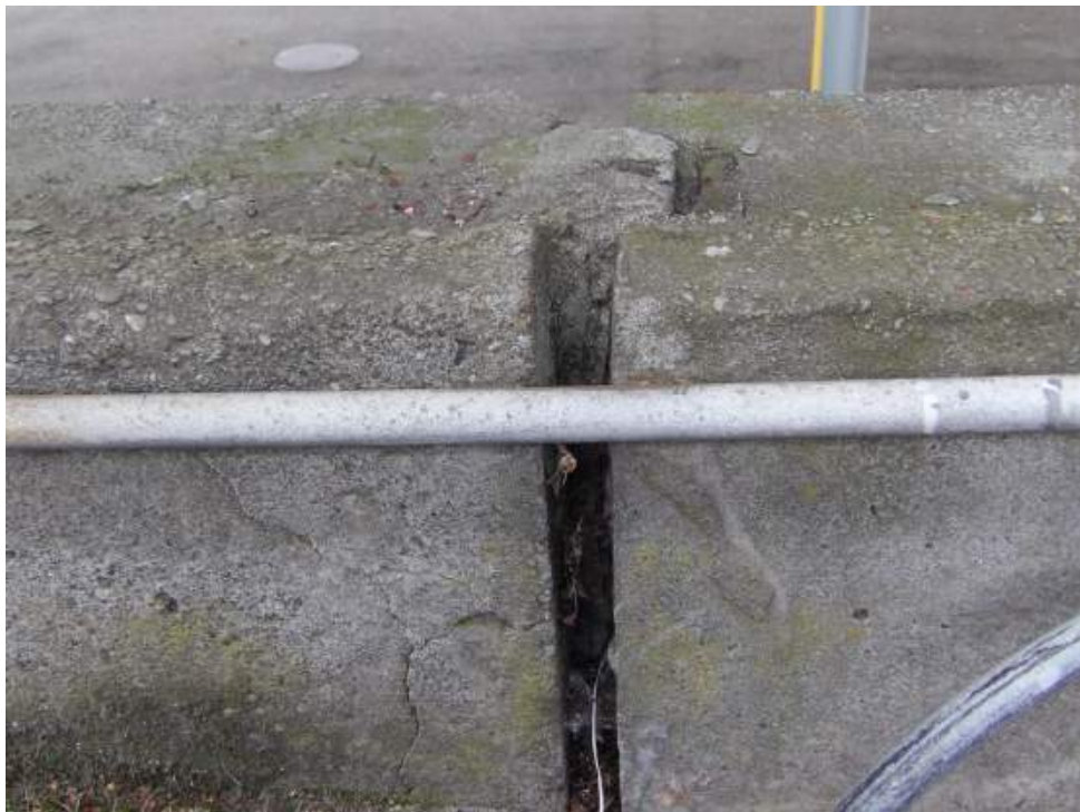
FIGURE F1B: CRACKING AND SPALLING IN FRONT BEARING CONCRETE WALL
