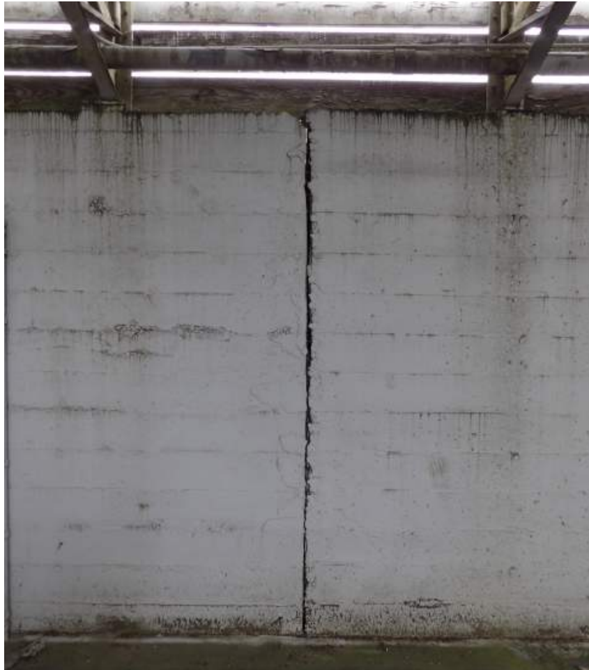
FIGURE F2B: MINOR SPALLING AT TOP OF WALL JOINT
