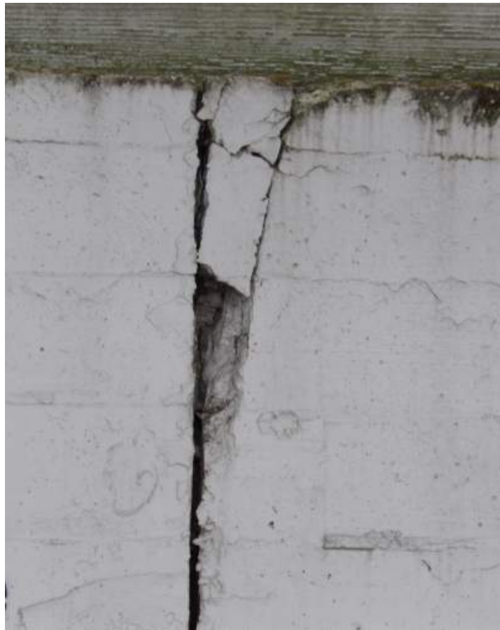
FIGURE F1D: SPALLING AT TOP OF WALL JOINT
