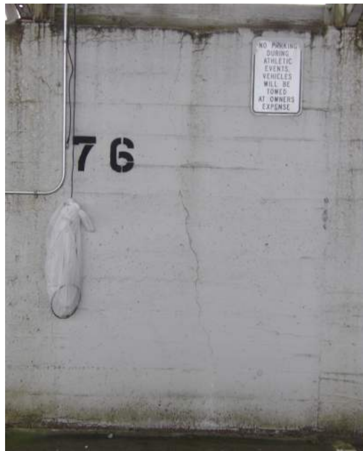
FIGURE F2E: MINOR VERTICAL CRACKING IN WALL (TYPICAL OF ENTIRE WALL)
