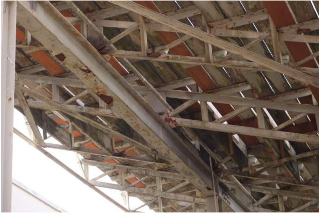
FIGURE S2H: TYPICAL SLIGHT CORROSION
