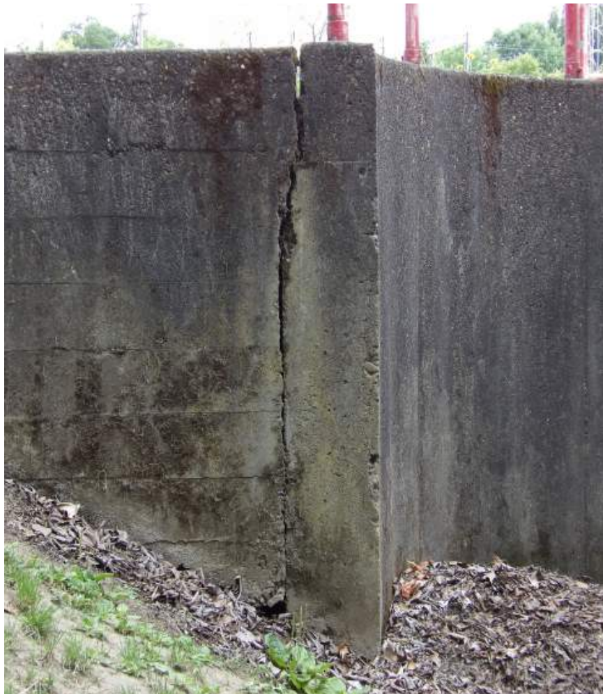
FIGURE F4A: CONCRETE WALL SEPARATION AT CORNER
