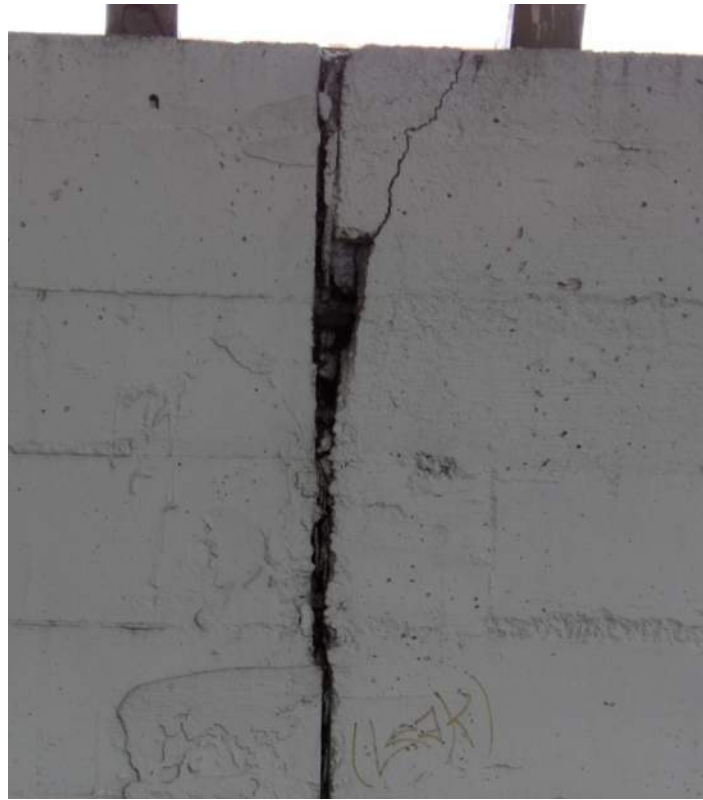
FIGURE F1C: CRACKING AND SPALLING IN FRONT BEARING CONCRETE WALL
