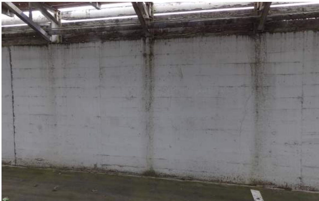
FIGURE F2C: MINOR VERTICAL CRACKING IN WALL (TYPICAL OF ENTIRE WALL)
