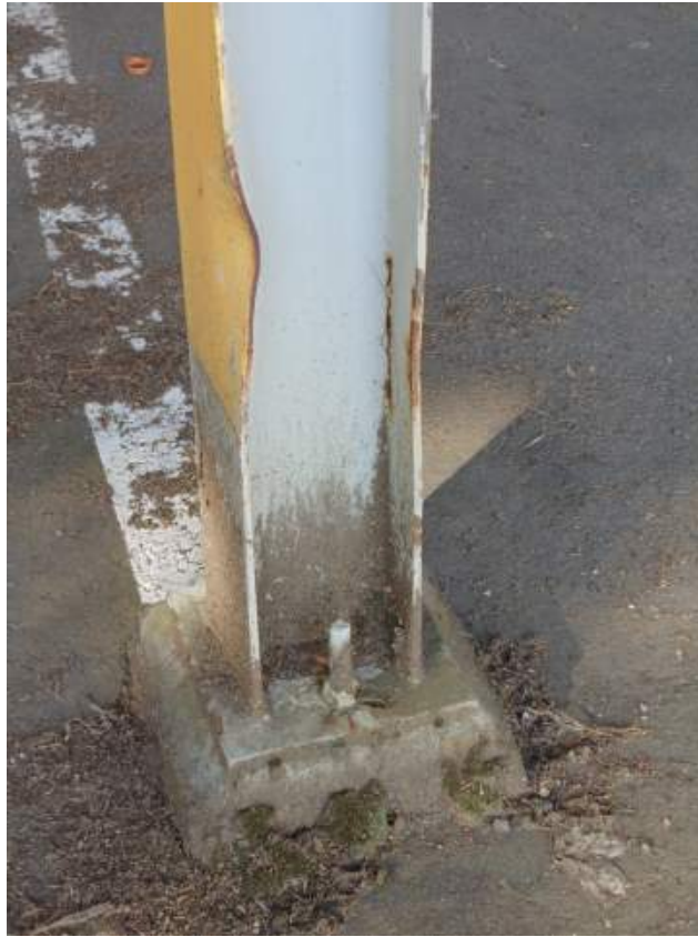
FIGURE S1A: STEEL COLUMN DAMAGE
