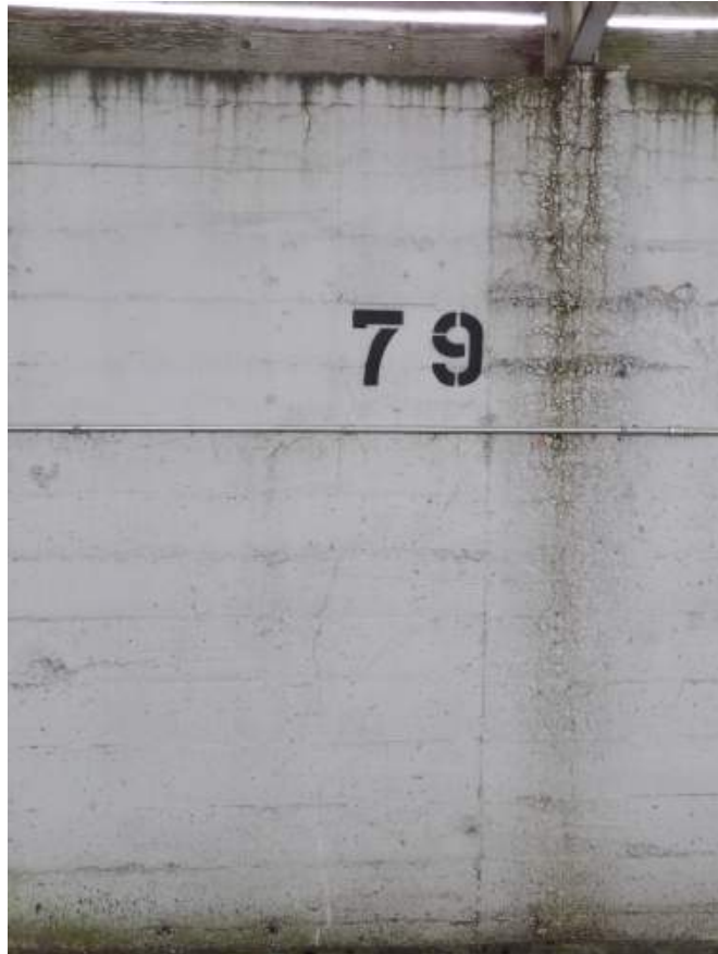
FIGURE F2A: MINOR CRACKING IN FRONT BEARING CONCRETE WALL (TYPICAL OF ENTIRE WALL)
