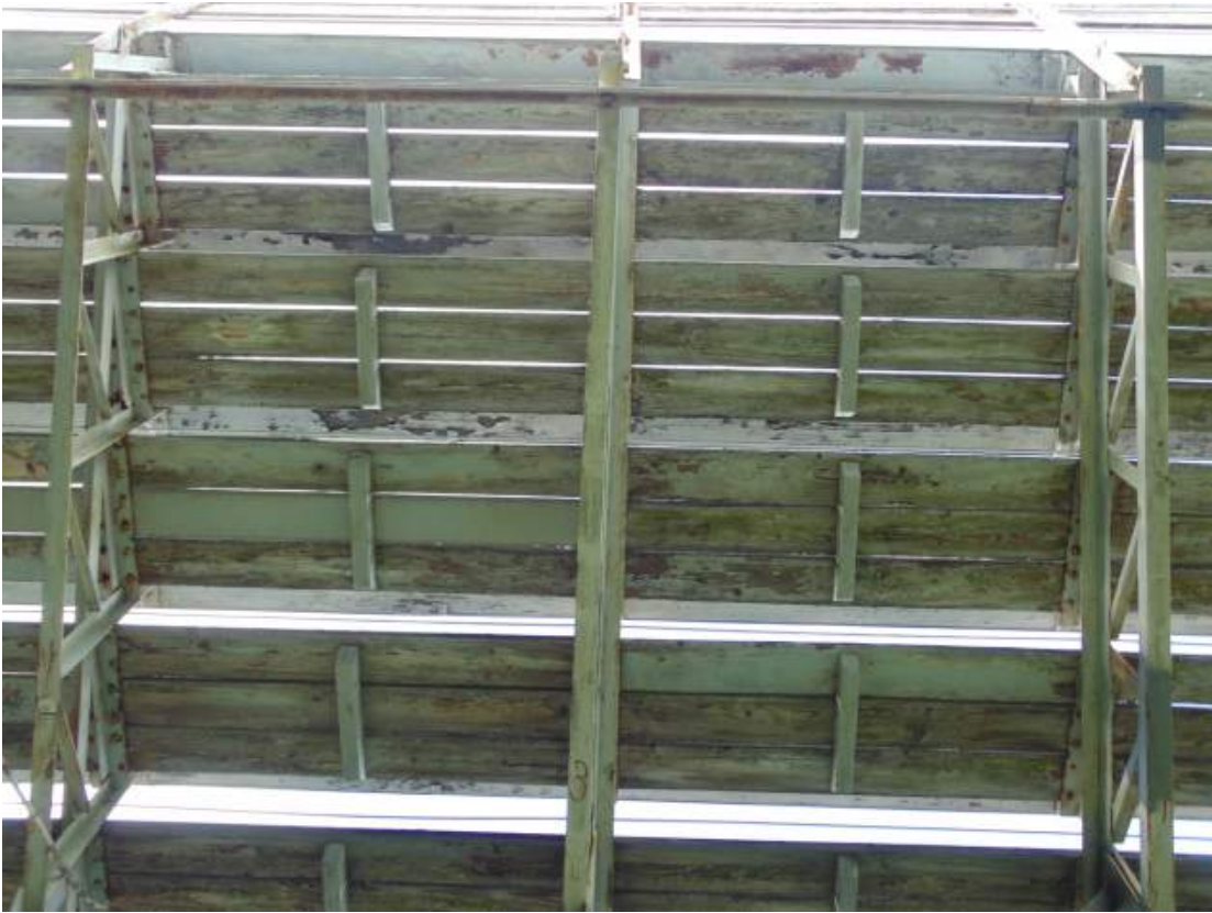
FIGURE S5C: BLEACHER BOARD STEEL SUPPORT RUSTING FROM TOP
