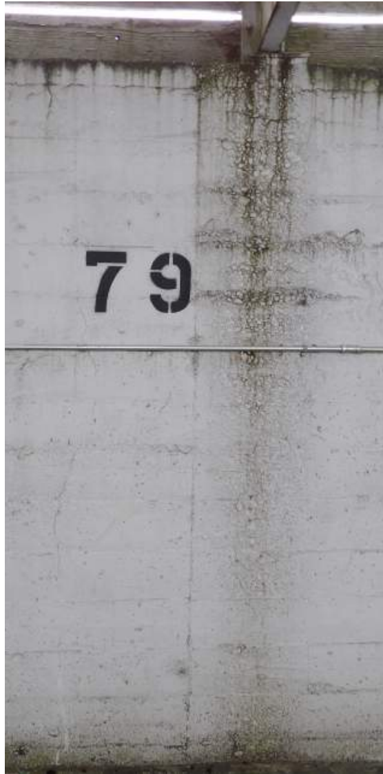
FIGURE F5A: CONCRETE EROSION DUE TO WATER
