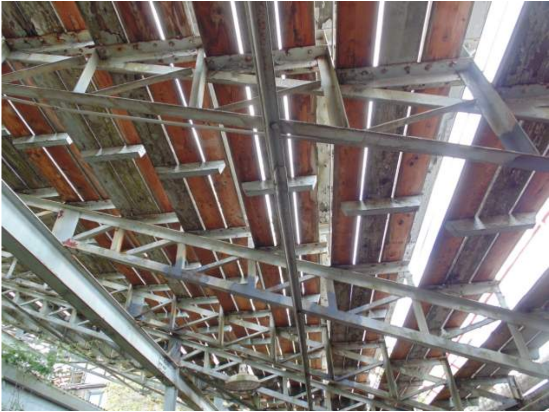
FIGURE S5A: BLEACHER BOARD STEEL SUPPORT RUSTING FROM TOP
