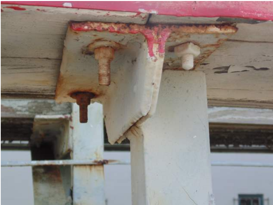
FIGURE S5B: BLEACHER BOARD STEEL SUPPORT RUSTING FROM TOP
