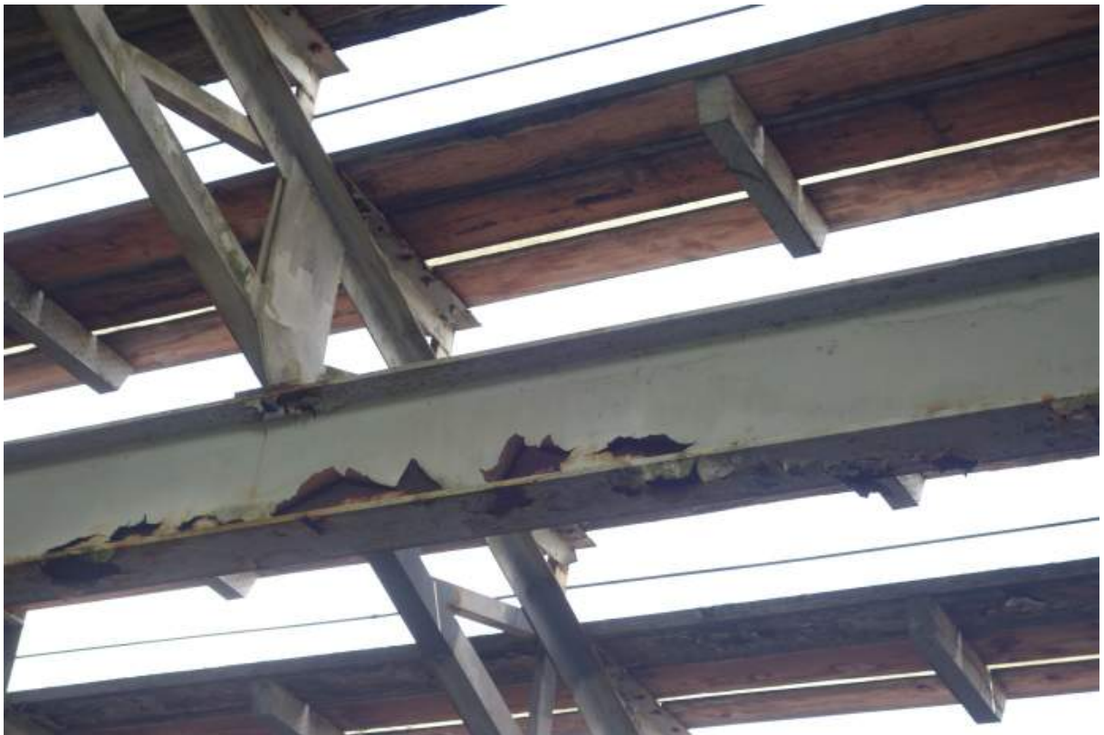
FIGURE S2G: TYPICAL SLIGHT CORROSION
