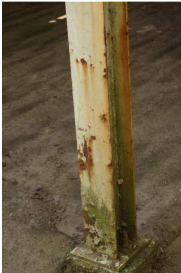
FIGURE S2E: TYPICAL SLIGHT CORROSION
