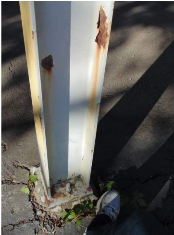
FIGURE S2D: TYPICAL SLIGHT CORROSION
