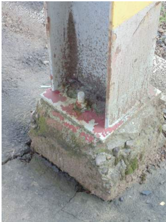
FIGURE S2A: TYPICAL SLIGHT CORROSION
