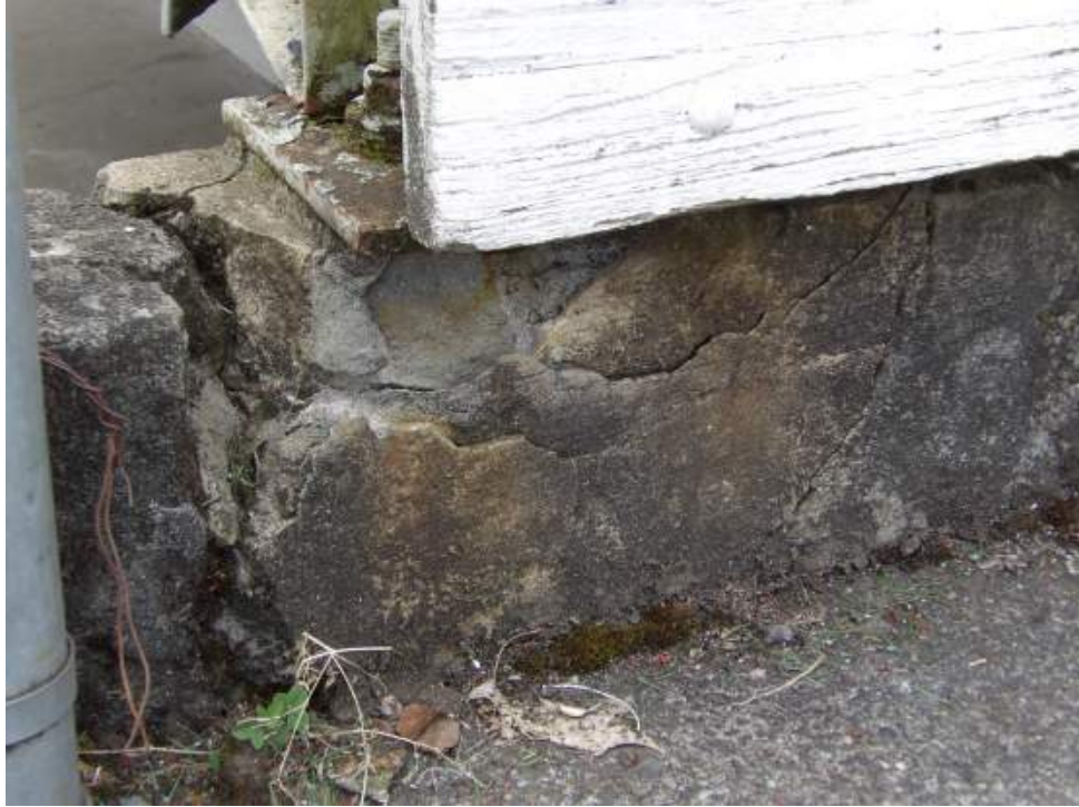
FIGURE F1A: CRACKING AND SPALLING IN FRONT BEARING CONCRETE WALL
