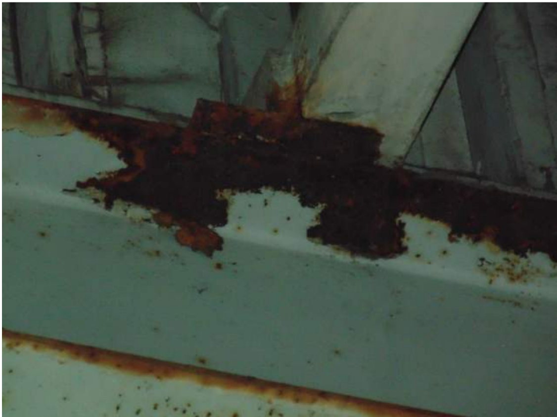
FIGURE S4C: SIGNIFICANT CORROSION ON STEEL BEAM ADDED FOR PRESSBOX
