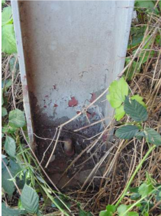
FIGURE S3B: SLIGHT CORROSION ON COLUMN ALONG WITH EMBEDDED DEBRIS
