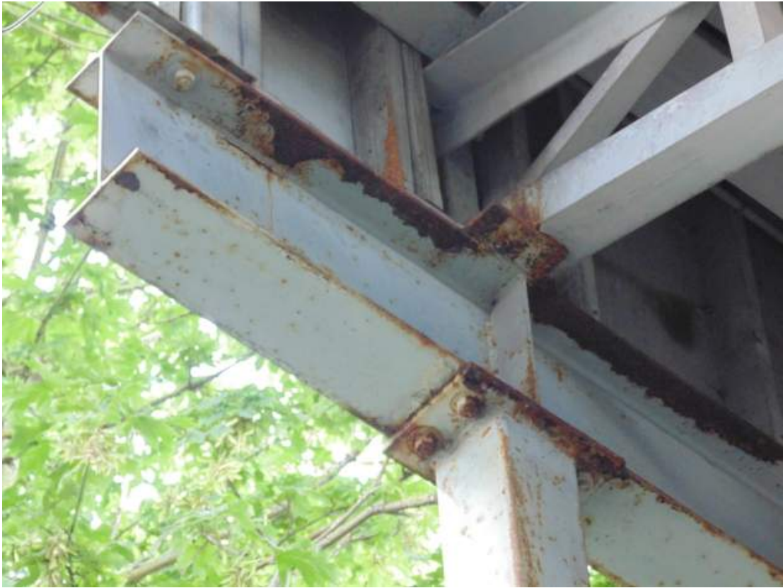
FIGURE S4B: SIGNIFICANT CORROSION ON STEEL BEAM ADDED FOR PRESSBOX
