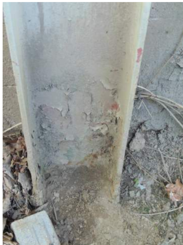
FIGURE S3C: SLIGHT CORROSION ON COLUMN ALONG WITH EMBEDDED DEBRIS
