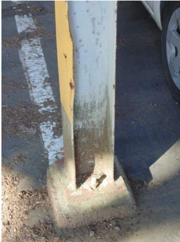
FIGURE S1C: STEEL COLUMN DAMAGE
