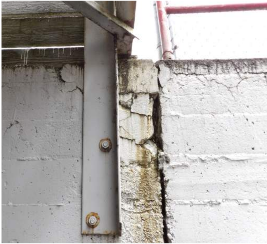
FIGURE F1E: CRACKING AND SPALLING AT TOP OF CONCRETE WALL
