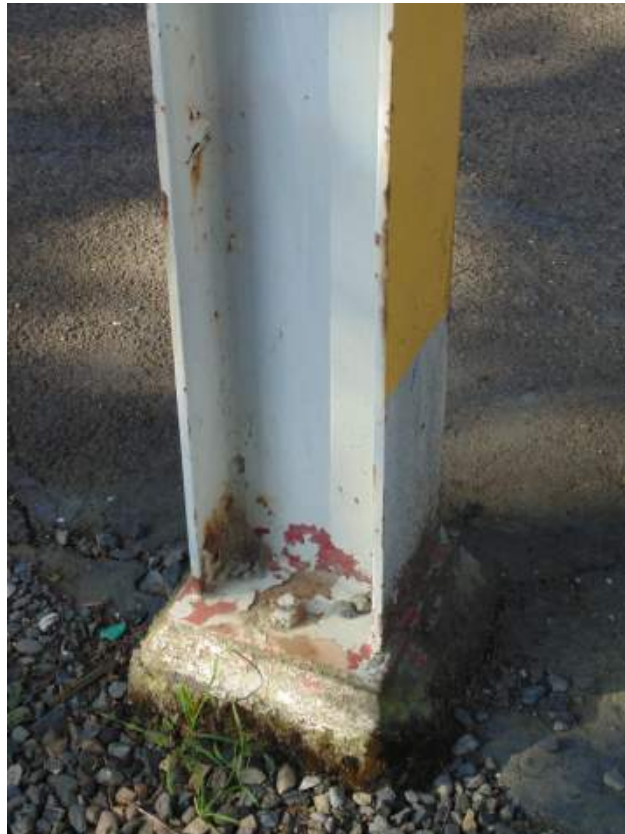
FIGURE S2C: TYPICAL SLIGHT CORROSION
