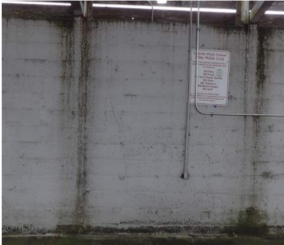
FIGURE F2D: MINOR VERTICAL CRACKING IN WALL (TYPICAL OF ENTIRE WALL)
