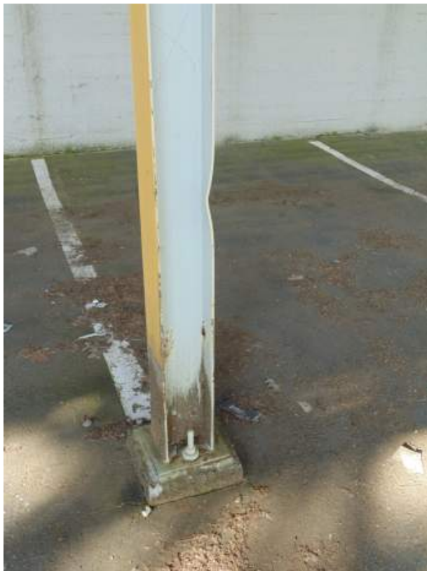
FIGURE S1B: STEEL COLUMN DAMAGE
