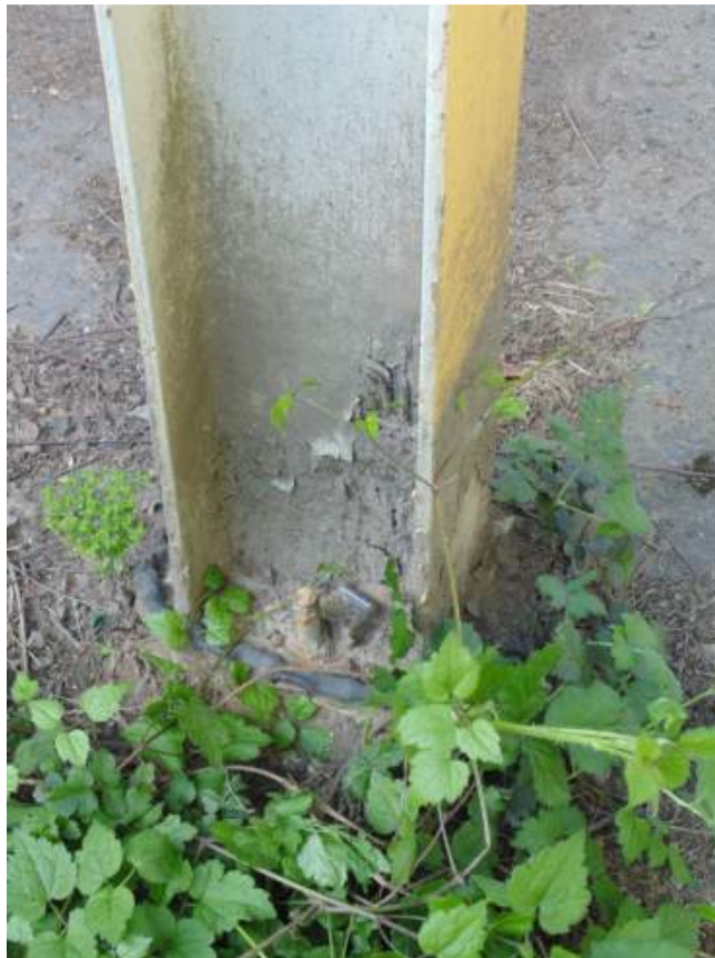
FIGURE S3A: SLIGHT CORROSION ON COLUMN ALONG WITH EMBEDDED DEBRIS
