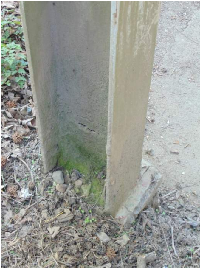
FIGURE S3D: SLIGHT CORROSION ON COLUMN ALONG WITH EMBEDDED DEBRIS
