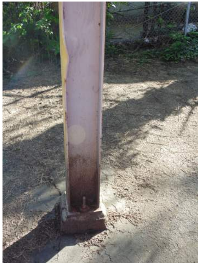
FIGURE S1D: STEEL COLUMN DAMAGE
