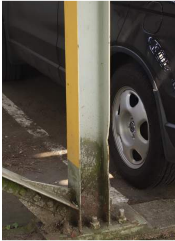
FIGURE S1E: STEEL COLUMN DAMAGE
