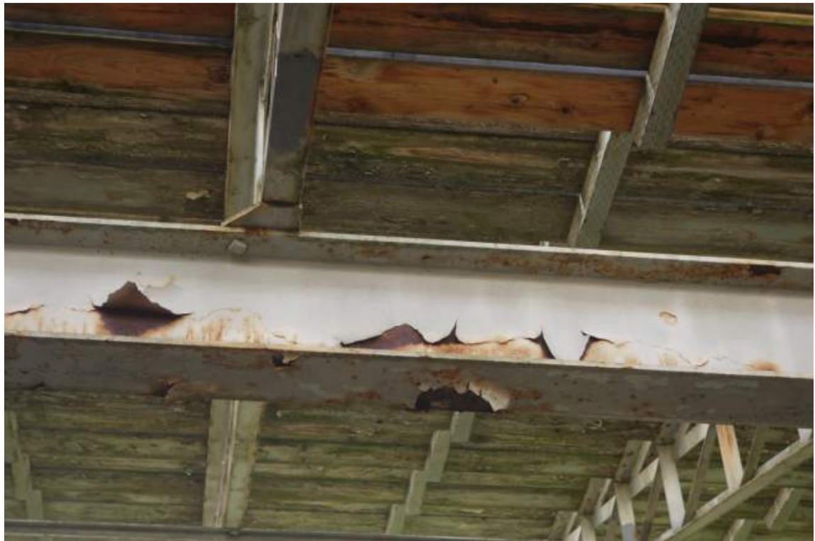
FIGURE S2F: TYPICAL SLIGHT CORROSION
