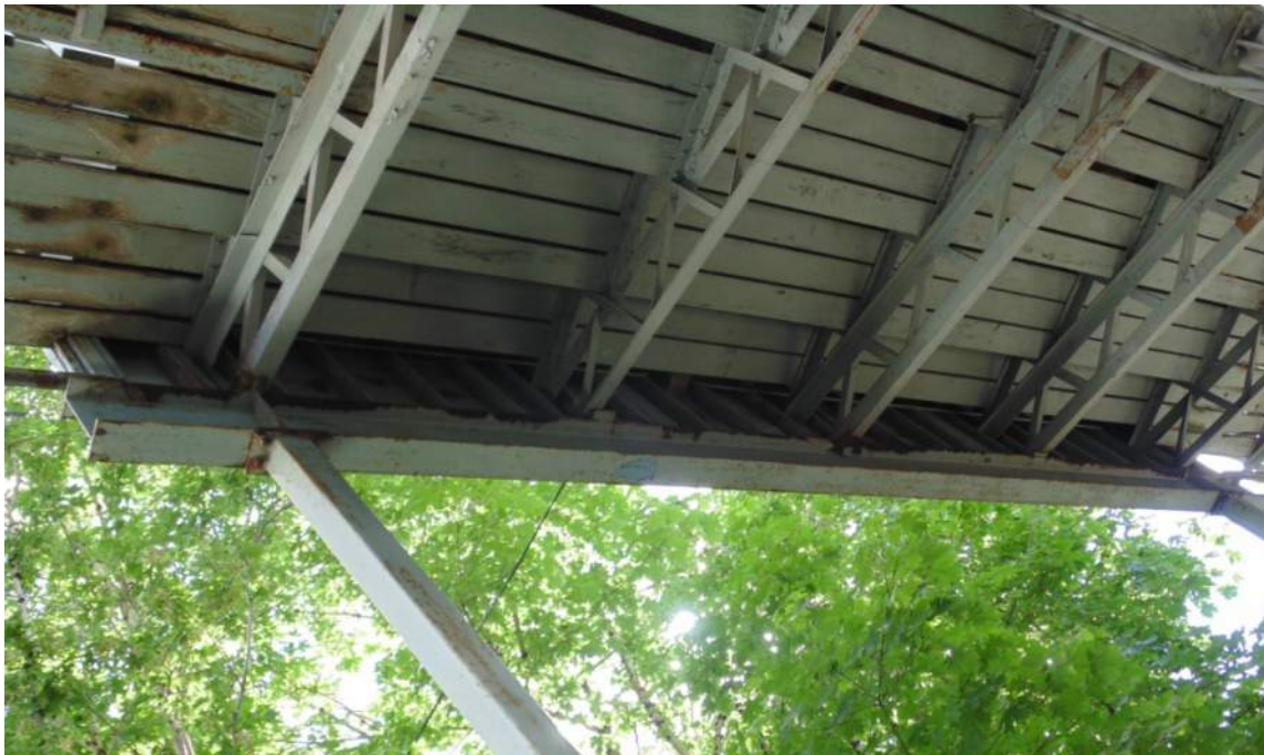
FIGURE S4A: SIGNIFICANT CORROSION ON STEEL BEAM ADDED FOR PRESSBOX
