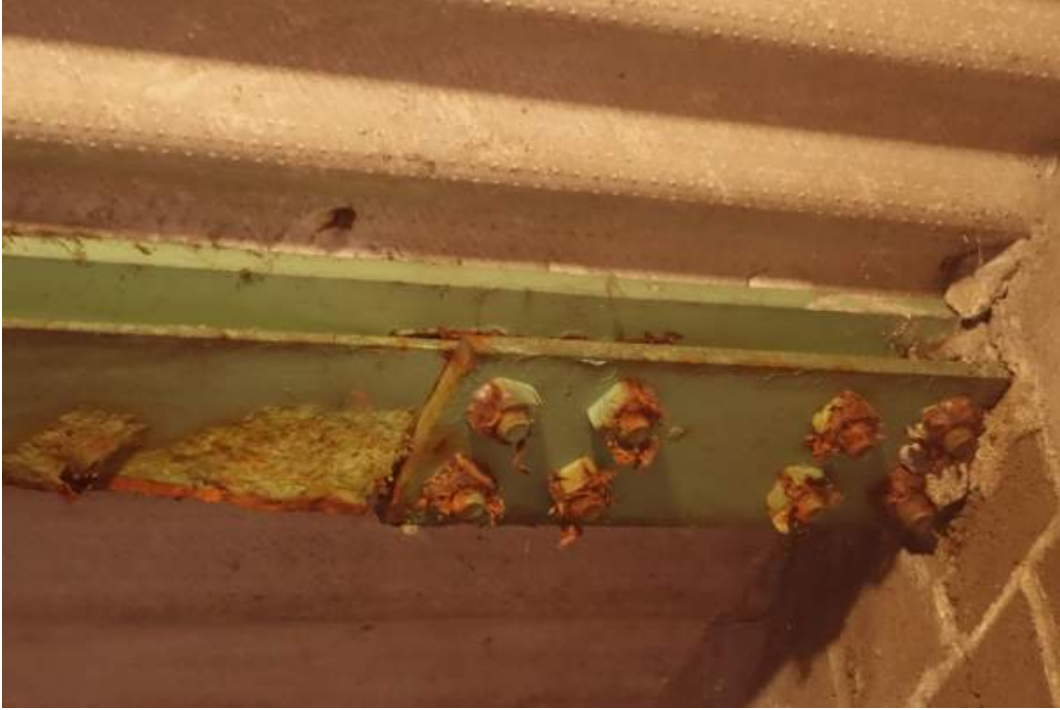
FIGURE S4I: SIGNIFICANT STEEL CORROSION AROUND AND IN MECHANICAL ROOM
