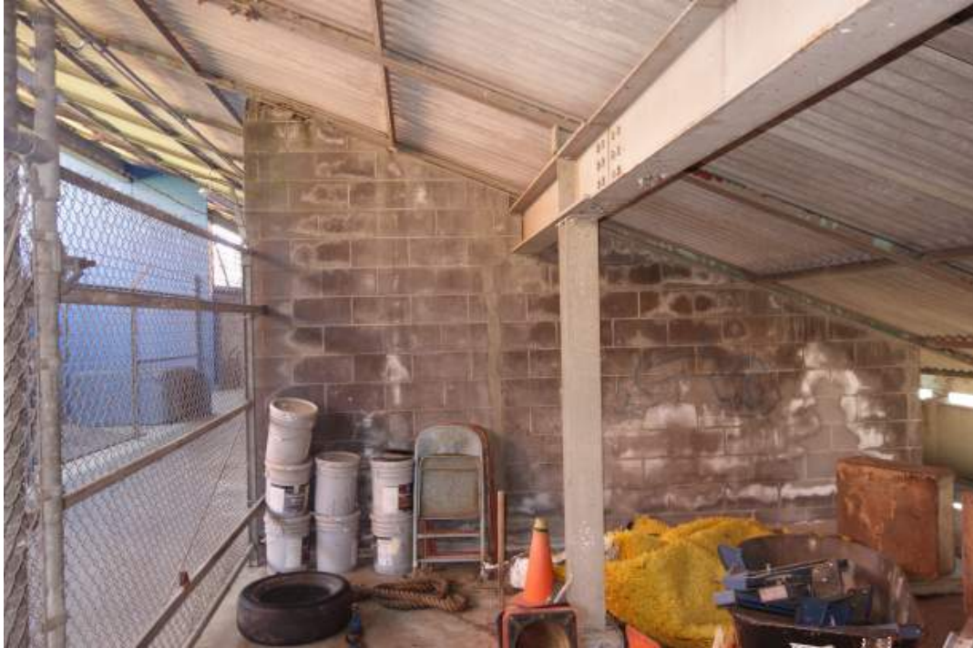
FIGURE S4Q: SIGNIFICANT STEEL CORROSION AROUND AND IN MECHANICAL ROOM
