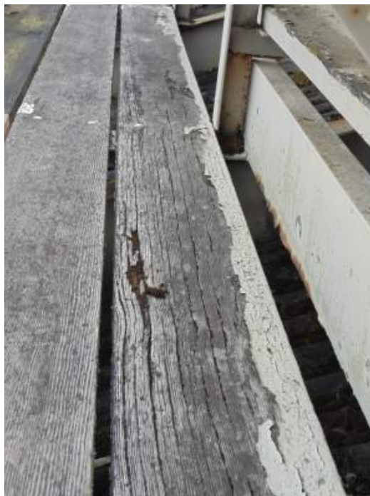
FIGURE B2A: DAMAGED / WEATHERED BLEACHER BOARDS
