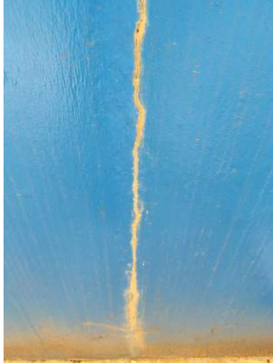
FIGURE F6C: VERTICAL CRACKS IN BACK RETAINING WALL (TYPICAL OF WALL)
