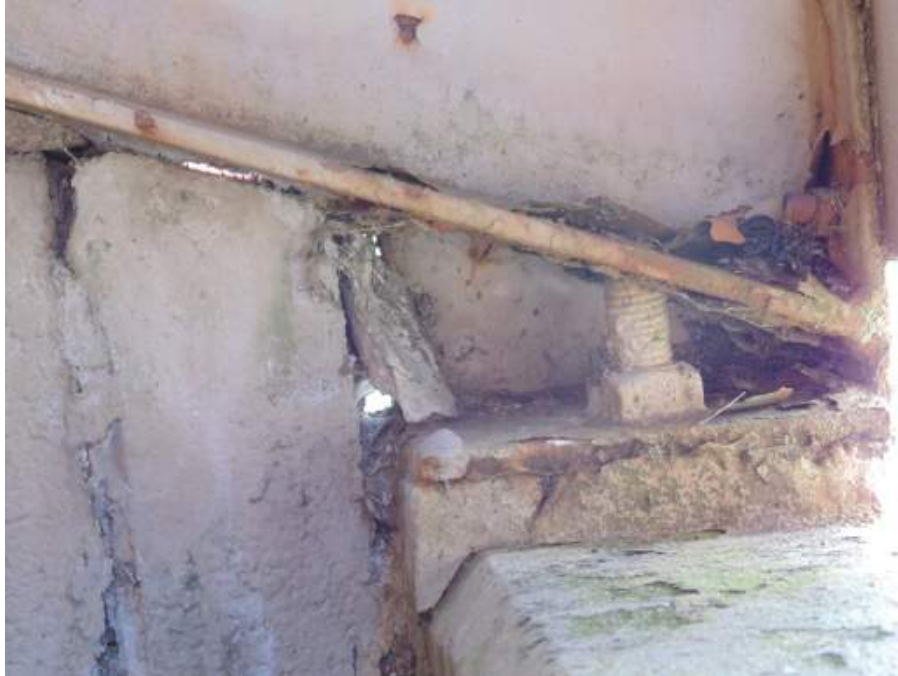
FIGURE S1A: GENERAL RUSTING OF THE STEEL STRUCTURE ABOVE AND BEYOND SURFACE RUSTING
