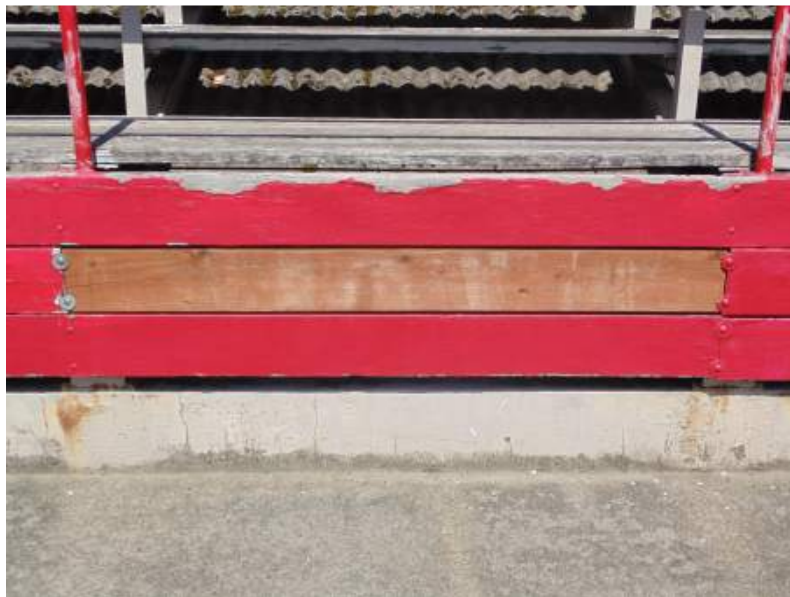
FIGURE F3A: MINOR CRACKING IN FRONT BEARING CONCRETE STEMWALL TYPICAL OF ENTIRE STEMWALL
