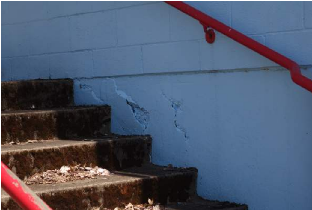
FIGURE F3C: MINOR CRACKING AND SPALLING IN CONCRETE WALL
