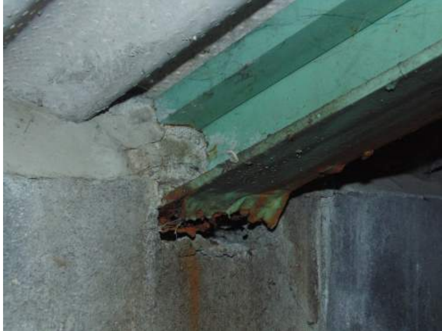
FIGURE S1C: GENERAL RUSTING OF STEEL STRUCTURE ABOVE AND BEYOND SURFACE RUSTING
