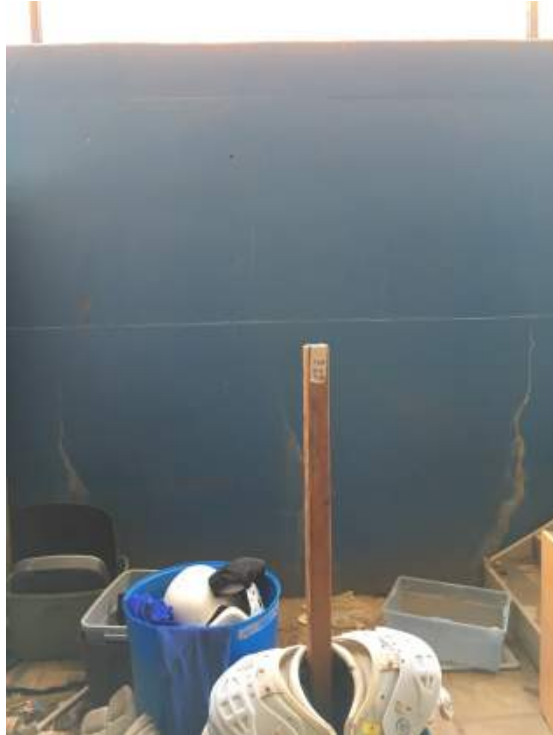
FIGURE F6A: VERTICAL CRACKS IN BACK RETAINING WALL (TYPICAL OF WALL)
