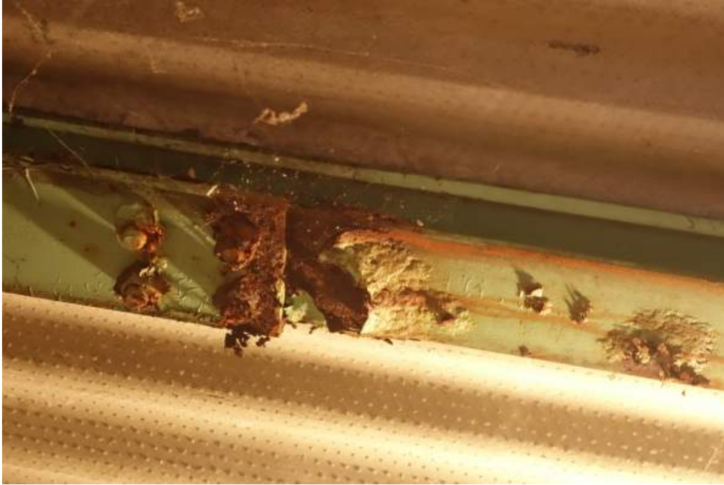
FIGURE S4G: SIGNIFICANT STEEL CORROSION AROUND AND IN MECHANICAL ROOM
