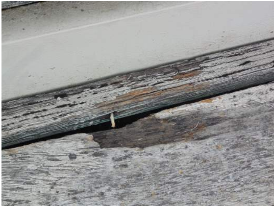
FIGURE B1B: SIGNIFICANTLY DAMAGED BLEACHER BOARDS
