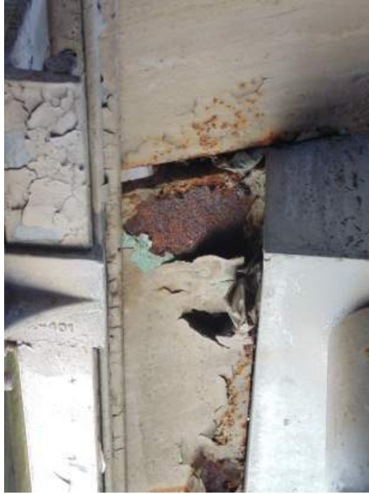
FIGURE S3A: SIGNIFICANT STEEL CORROSION AT CENTER GRANDSTAND BEAM
