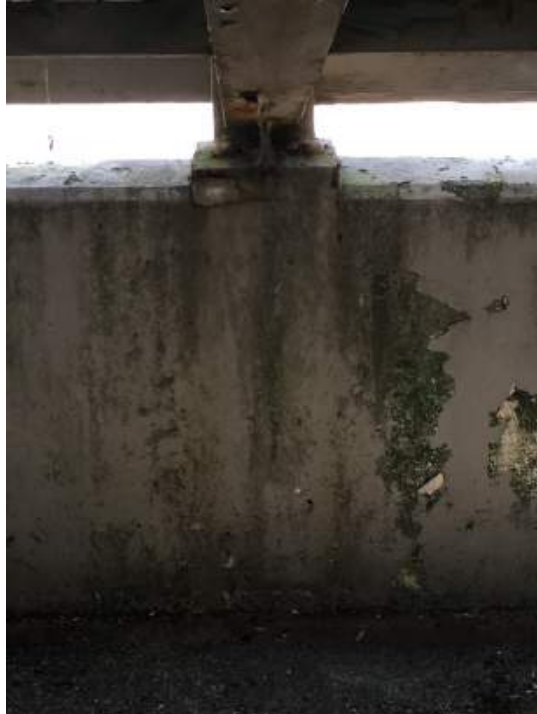
FIGURE F5C: PORTION OF NON-SHRINK GROUT BENEATH BASE PLATE IS DETERIORATING
