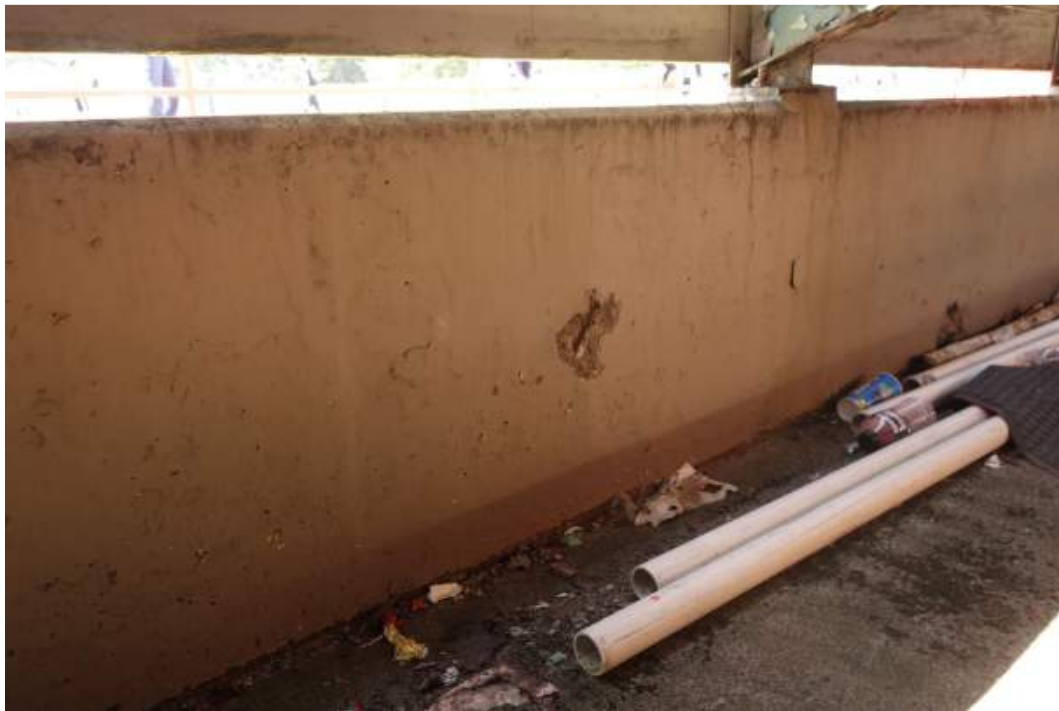
FIGURE F4B: SPALLING IN STEMWALL WITH REBAR EXPOSED
