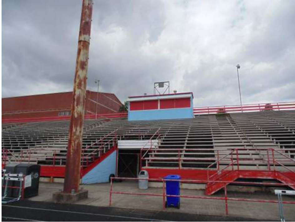
FIGURE R1A: LARGE SPACE BETWEEN RAILING AND BLEACHERS
