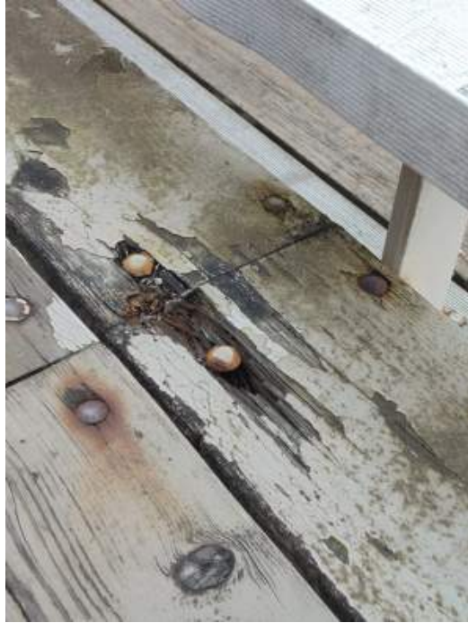
FIGURE B6A: SIGNIFICANT DAMAGE AT BLEACHER BOARD CONNECTION
