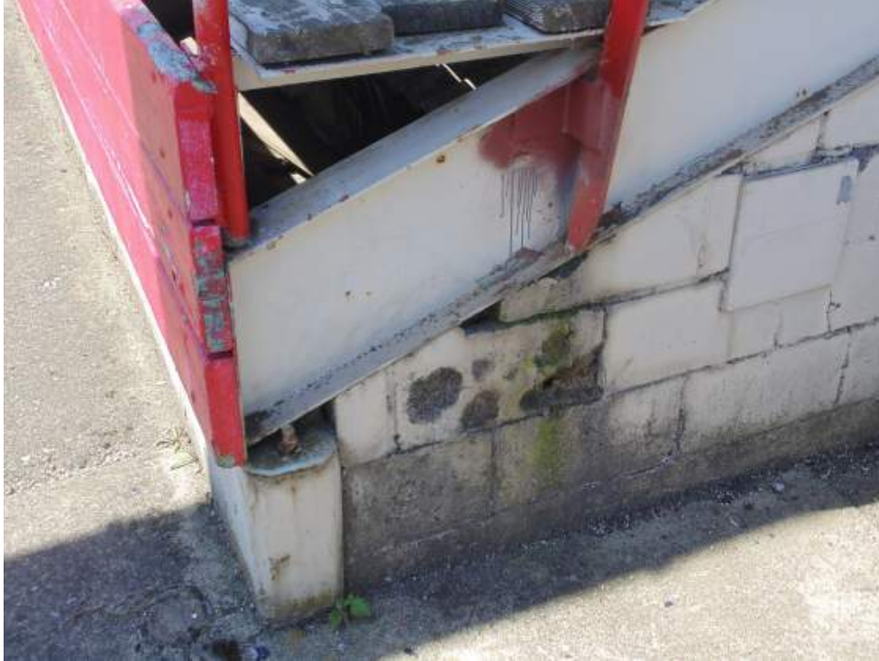
FIGURE F1A: DETERIORATION OF CMU
