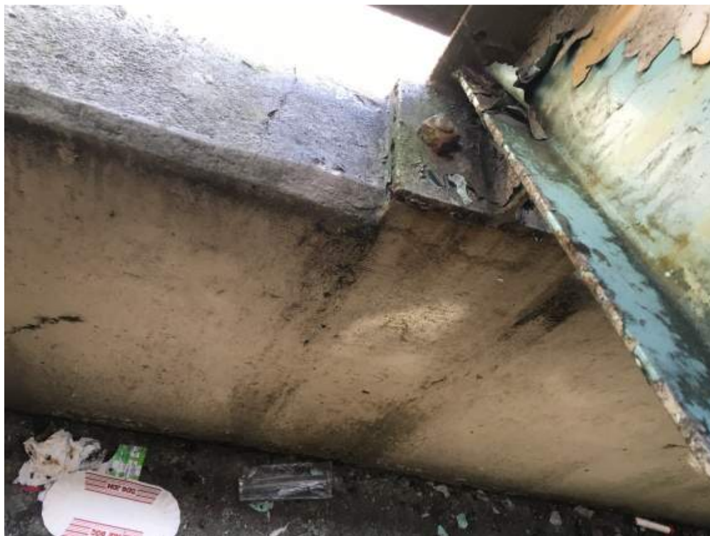
FIGURE S4V: SIGNIFICANT STEEL CORROSION AROUND AND IN MECHANICAL ROOM
