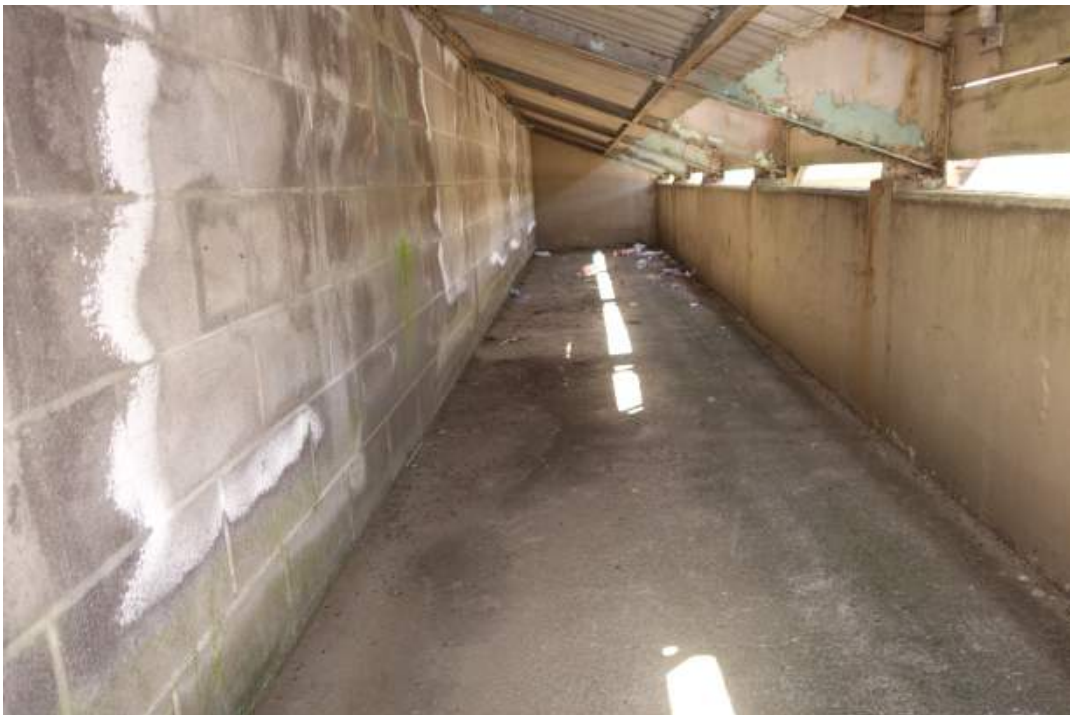
FIGURE S4T: SIGNIFICANT STEEL CORROSION AROUND AND IN MECHANICAL ROOM
