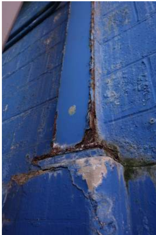
FIGURE S2A: SIGNIFICANT STEEL CORROSION AT STEEL COLUMN WITHIN CMU WALL
