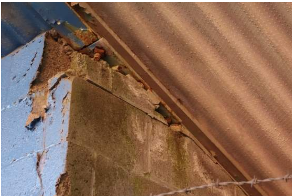
FIGURE S4D: SIGNIFICANT STEEL CORROSION AROUND AND IN MECHANICAL ROOM
