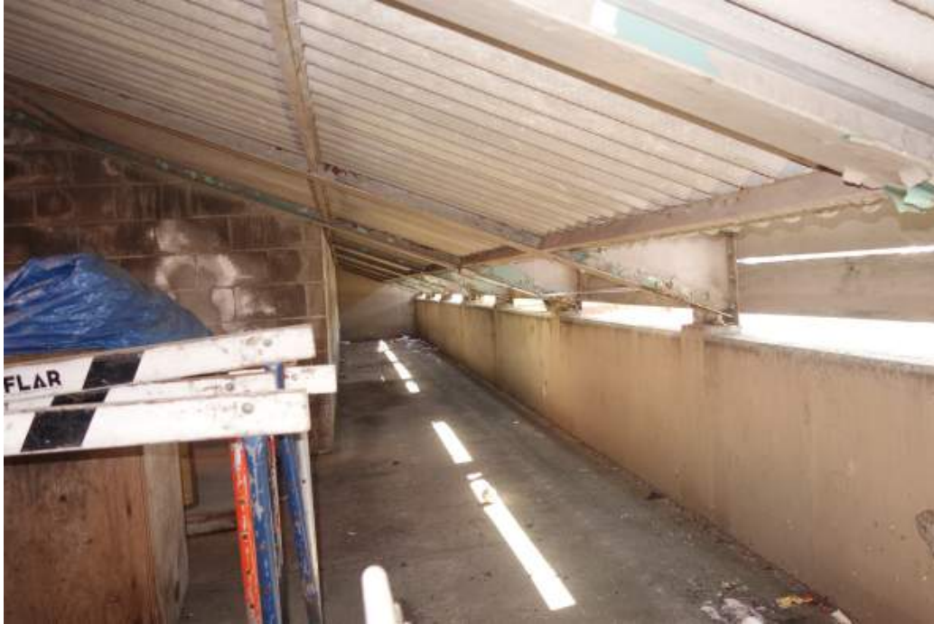
FIGURE S4O: SIGNIFICANT STEEL CORROSION AROUND AND IN MECHANICAL ROOM
