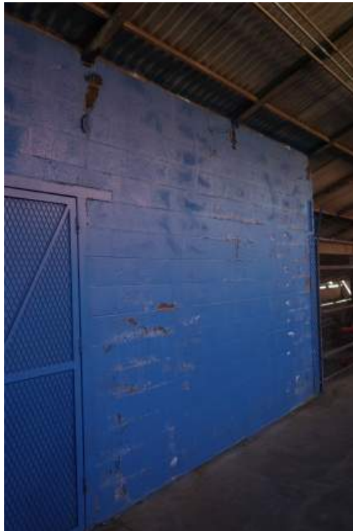
FIGURE S4B: SIGNIFICANT STEEL CORROSION AROUND AND IN MECHANICAL ROOM
