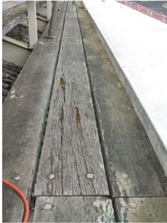
FIGURE B1E: SIGNIFICANTLY DAMAGED BLEACHER BOARDS
