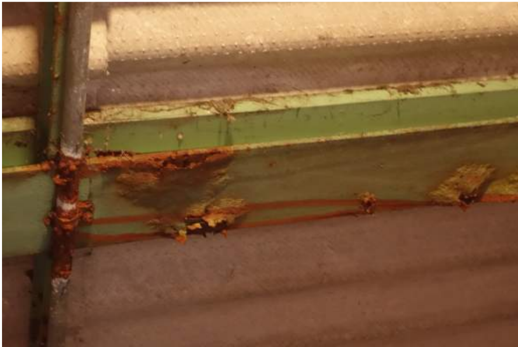
FIGURE S4H: SIGNIFICANT STEEL CORROSION AROUND AND IN MECHANICAL ROOM
