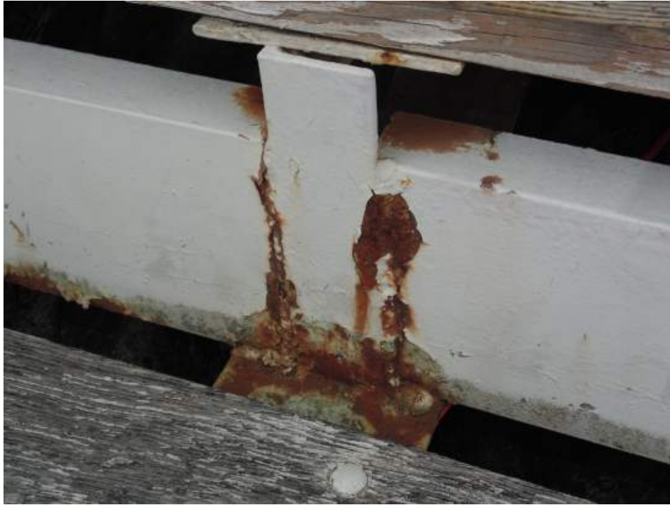
FIGURE S5E: BLEACHER BOARD STEEL SUPPORT RUSTING FROM TOP
