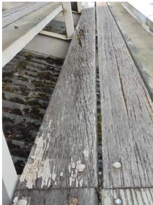
FIGURE B1F: SIGNIFICANTLY DAMAGED BLEACHER BOARDS
