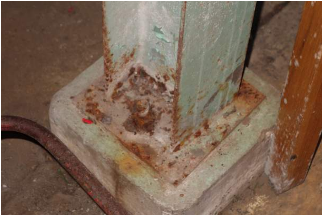
FIGURE S4J: SIGNIFICANT STEEL CORROSION AROUND AND IN MECHANICAL ROOM
