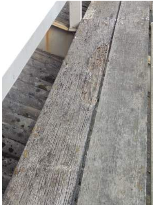
FIGURE B1: SIGNIFICANTLY DAMAGED BLEACHER BOARDS
