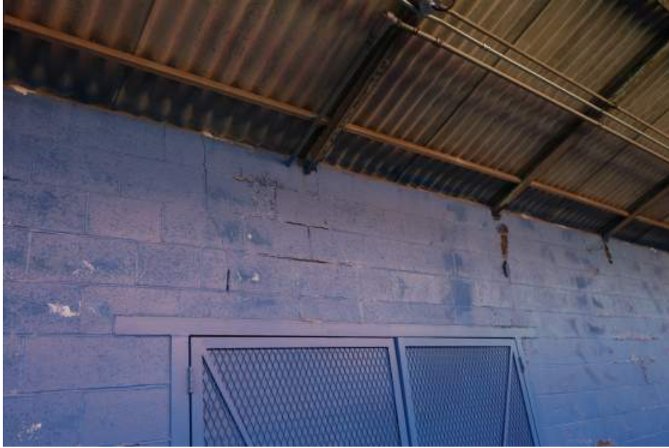
FIGURE S4A: SIGNIFICANT STEEL CORROSION AROUND AND IN MECHANICAL ROOM
