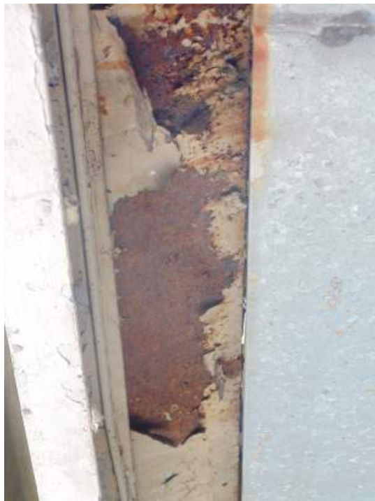
FIGURE S3B: SIGNIFICANT STEEL CORROSION AT CENTER GRANDSTAND BEAM
