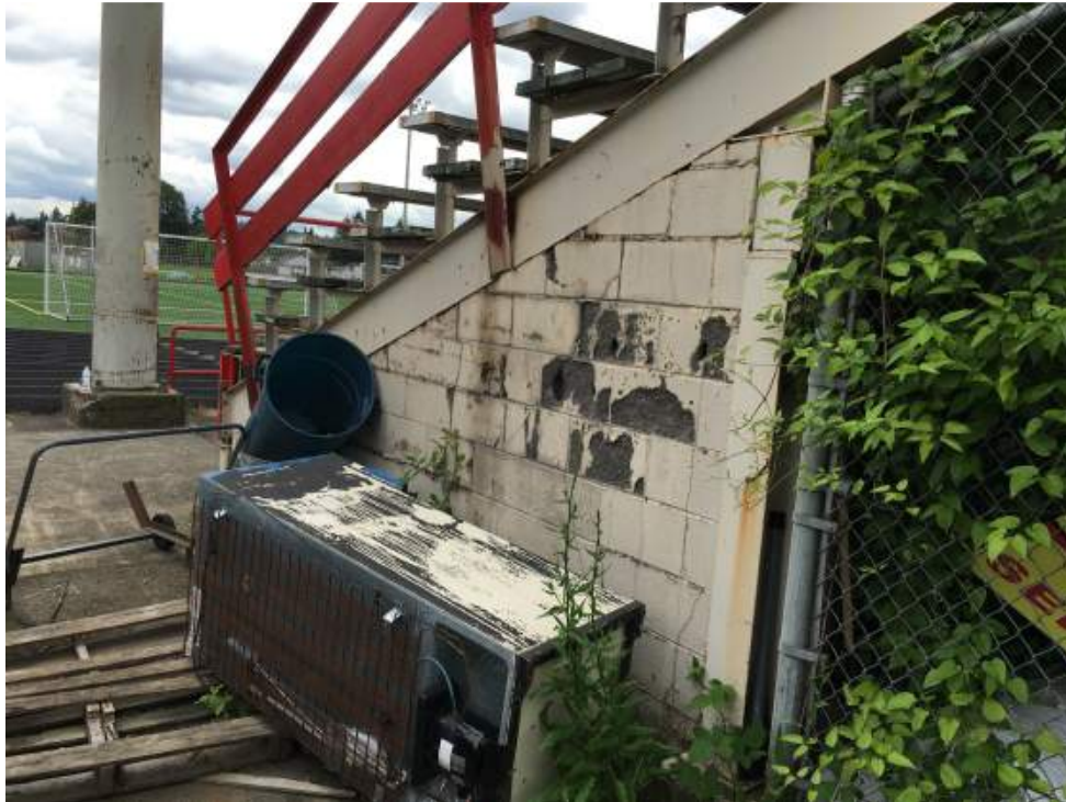
FIGURE F1B: DETERIORATION OF CMU
