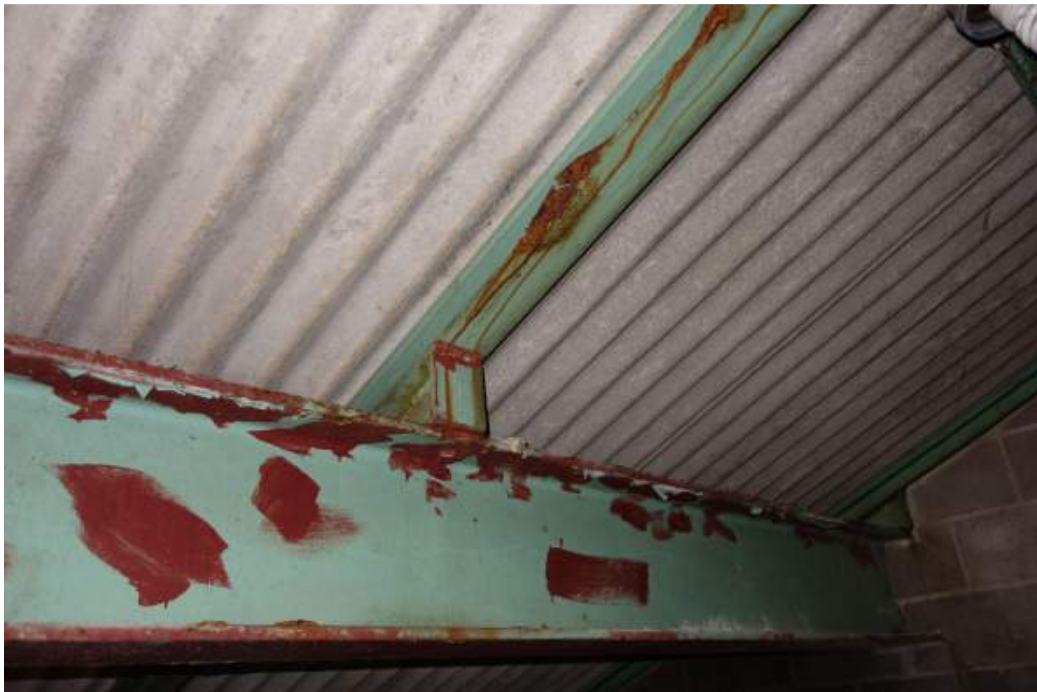
FIGURE S4N: SIGNIFICANT STEEL CORROSION AROUND AND IN MECHANICAL ROOM
