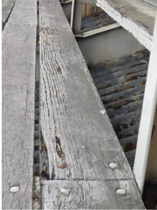
FIGURE B1C: SIGNIFICANTLY DAMAGED BLEACHER BOARDS
