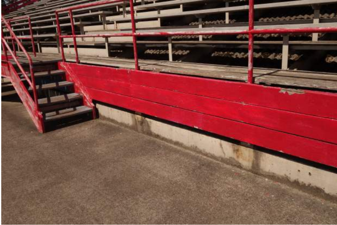
FIGURE F4A: CRACKING AND SPALLING IN FRONT BEARING CONCRETE STEMWALL
