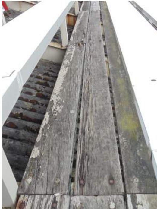
FIGURE B1G: SIGNIFICANTLY DAMAGED BLEACHER BOARDS
