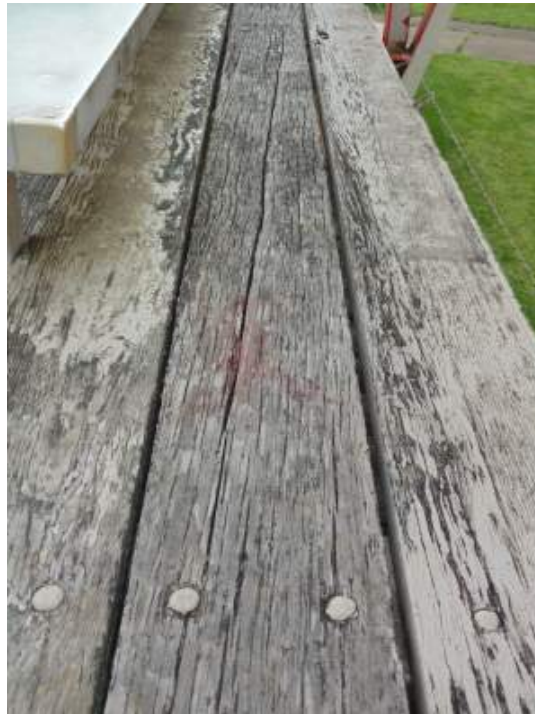
FIGURE B1D: SIGNIFICANTLY DAMAGED BLEACHER BOARDS
