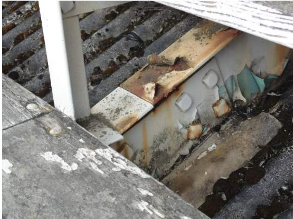
FIGURE S5D: BLEACHER BOARD STEEL SUPPORT RUSTING FROM TOP
