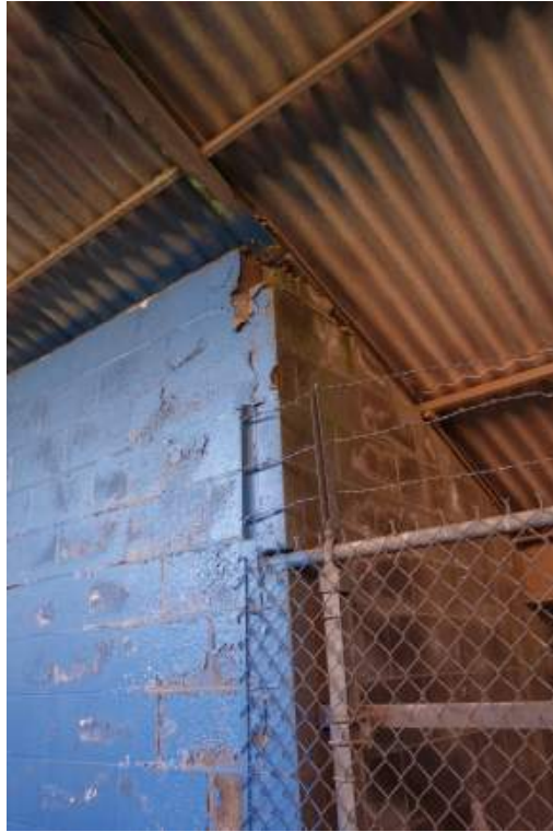
FIGURE S4C: SIGNIFICANT STEEL CORROSION AROUND AND IN MECHANICAL ROOM
