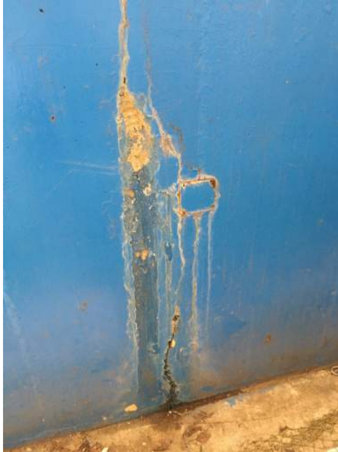
FIGURE F7D: SPALLING AND CRACKING
