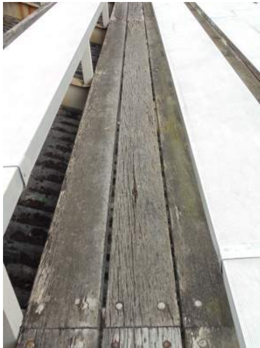
FIGURE B2E: DAMAGED / WEATHERED BLEACHER BOARDS
