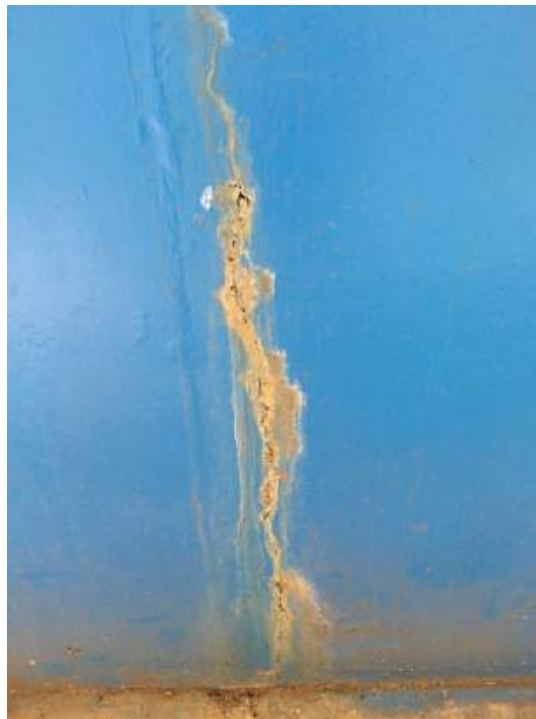
FIGURE F7C: SPALLING AND CRACKING
