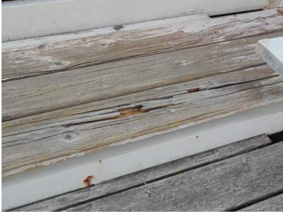
FIGURE B1A: SIGNIFICANTLY DAMAGED BLEACHER BOARDS
