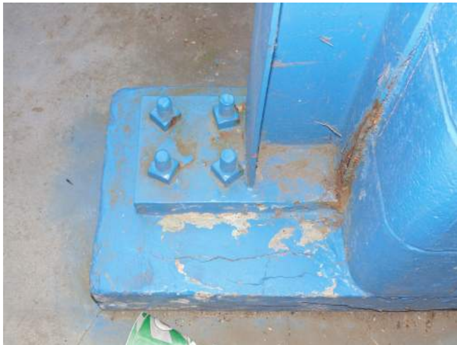
FIGURE S1B: GENERAL RUSTING OF STEEL STRUCTURE ABOVE AND BEYOND SURFACE RUSTING
