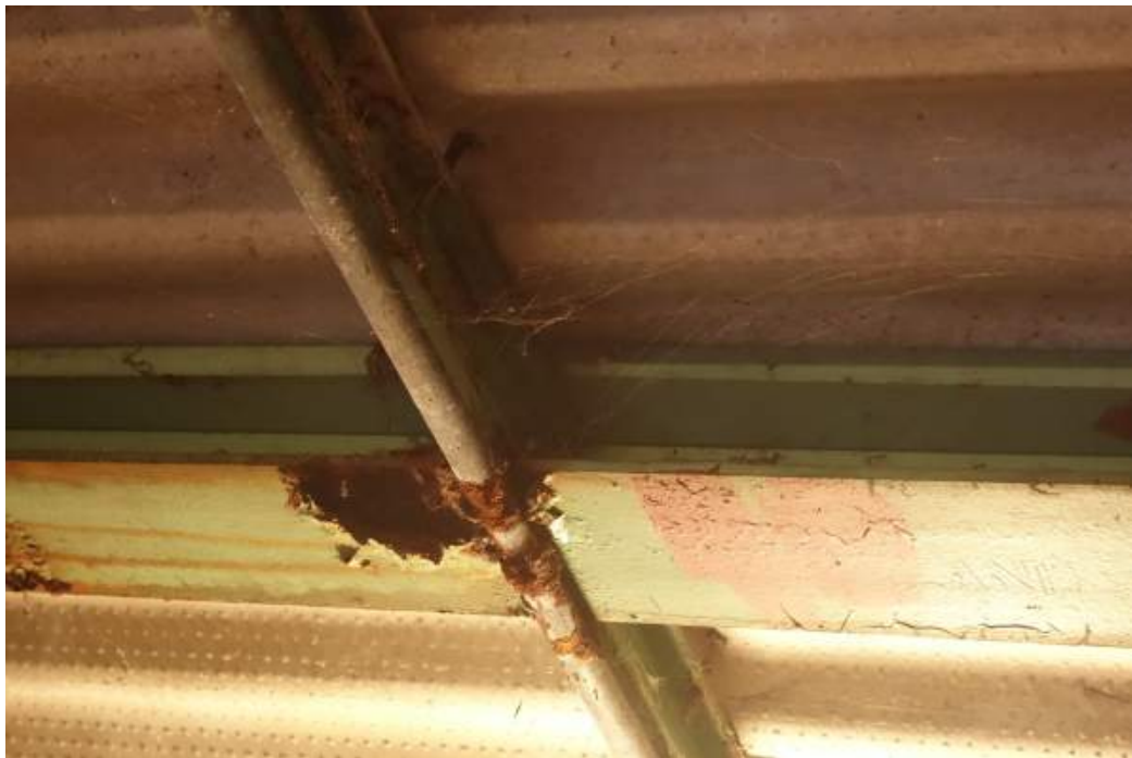
FIGURE S4F: SIGNIFICANT STEEL CORROSION AROUND AND IN MECHANICAL ROOM
