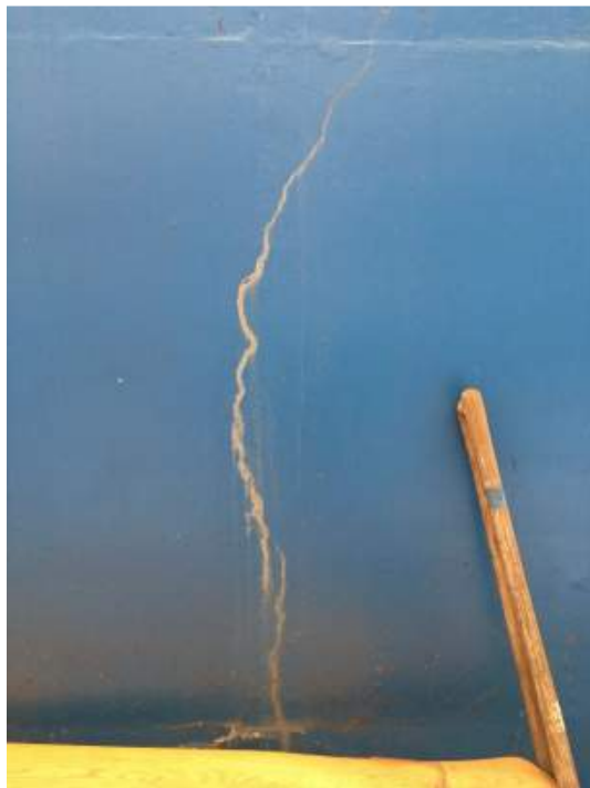
FIGURE F6B: VERTICAL CRACKS IN BACK RETAINING WALL (TYPICAL OF WALL)
