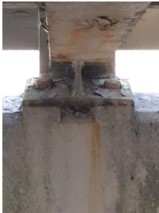
FIGURE F5D: PORTION OF NON-SHRINK GROUT BENEATH BASE PLATE IS DETERIORATING
