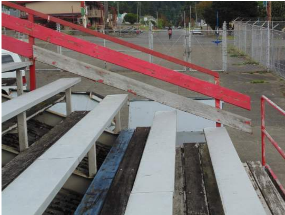
FIGURE R1C: LARGE SPACE BETWEEN RAILING AND BLEACHERS
