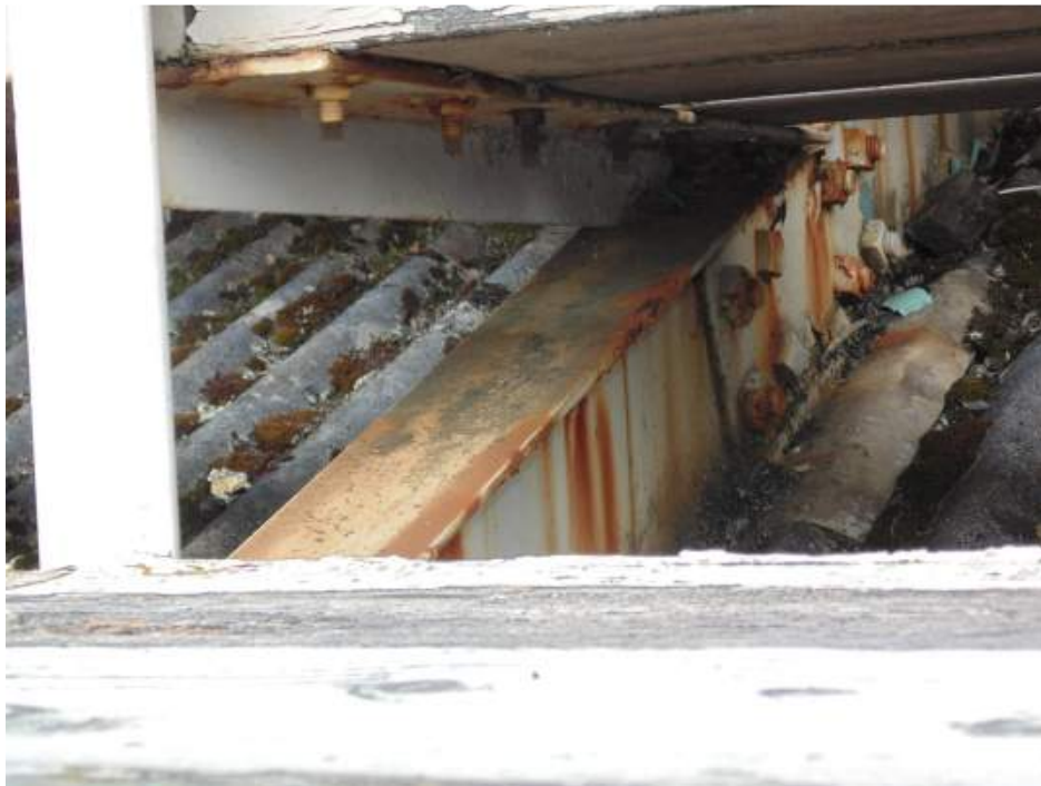
FIGURE S5F: BLEACHER BOARD STEEL SUPPORT RUSTING FROM TOP
