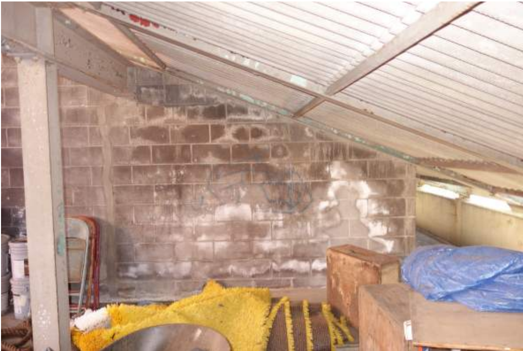
FIGURE S4P: SIGNIFICANT STEEL CORROSION AROUND AND IN MECHANICAL ROOM
