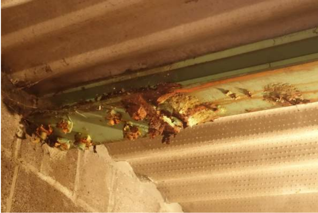
FIGURE S4E: SIGNIFICANT STEEL CORROSION AROUND AND IN MECHANICAL ROOM
