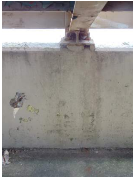
FIGURE F5B: PORTION ON NON-SHRINK GROUT BENEATH BASE PLATE IS DETERIORATING
