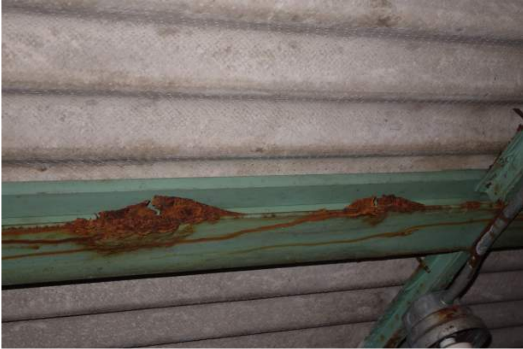
FIGURE S4K: SIGNIFICANT STEEL CORROSION AROUND AND IN MECHANICAL ROOM
