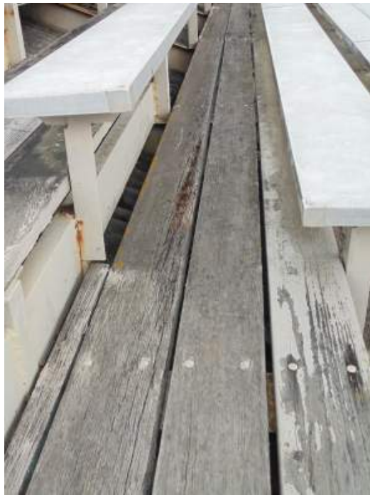
FIGURE B1H: SIGNIFICANTLY DAMAGED BLEACHER BOARDS
