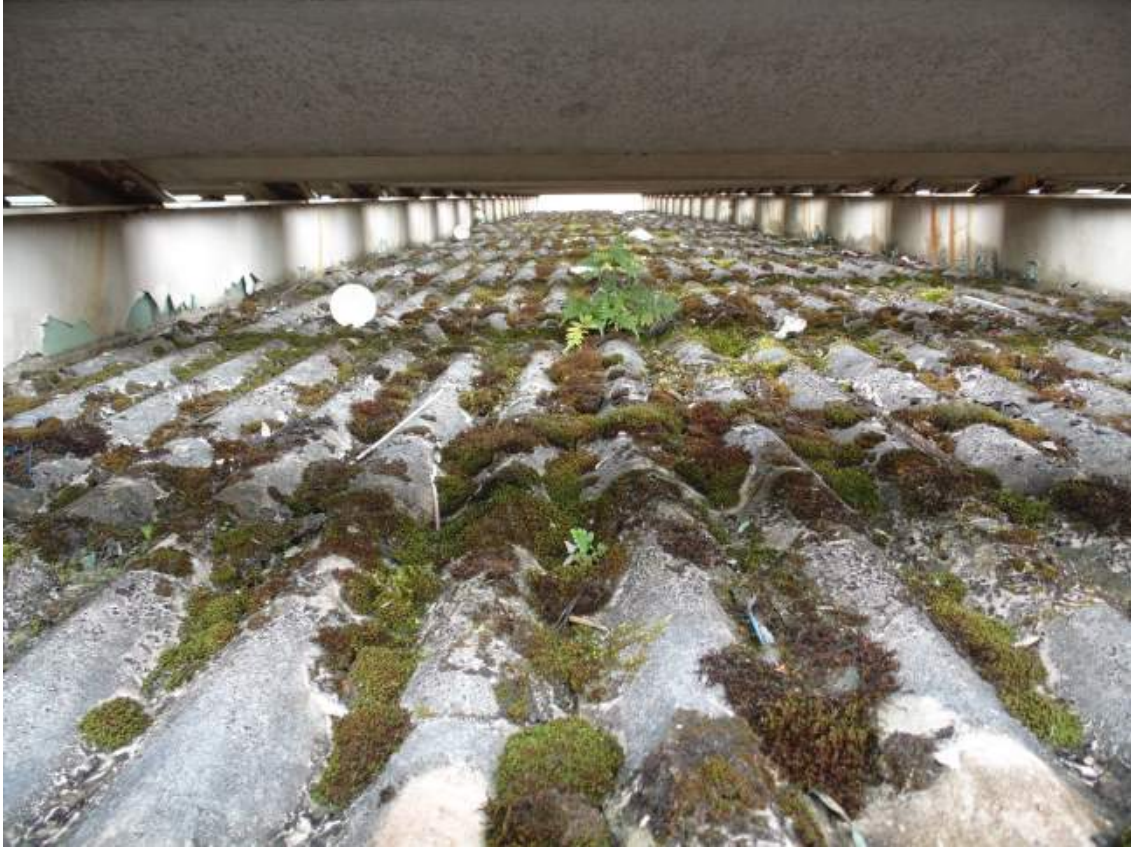
FIGURE S6A: HEAVY MOSS GROWTH ON CORRUGATED SOFFIT DECK
