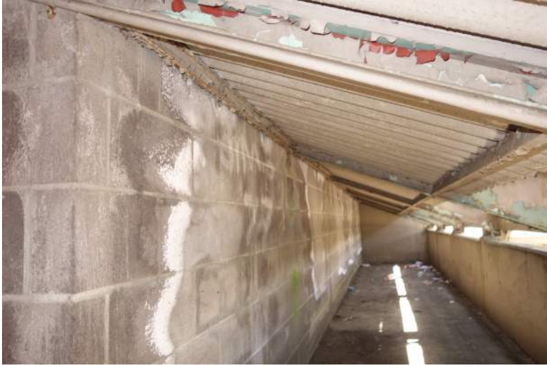
FIGURE S4S: SIGNIFICANT STEEL CORROSION AROUND AND IN MECHANICAL ROOM
