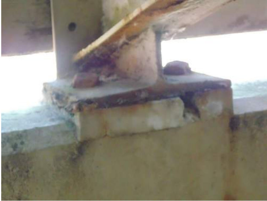
FIGURE F5A: PORTION ON NON-SHRINK GROUT BENEATH BASE PLATE IS DETERIORATING
