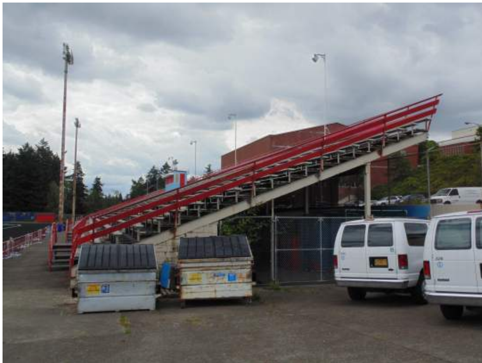
FIGURE R1B: LARGE SPACE BETWEEN RAILING AND BLEACHERS
