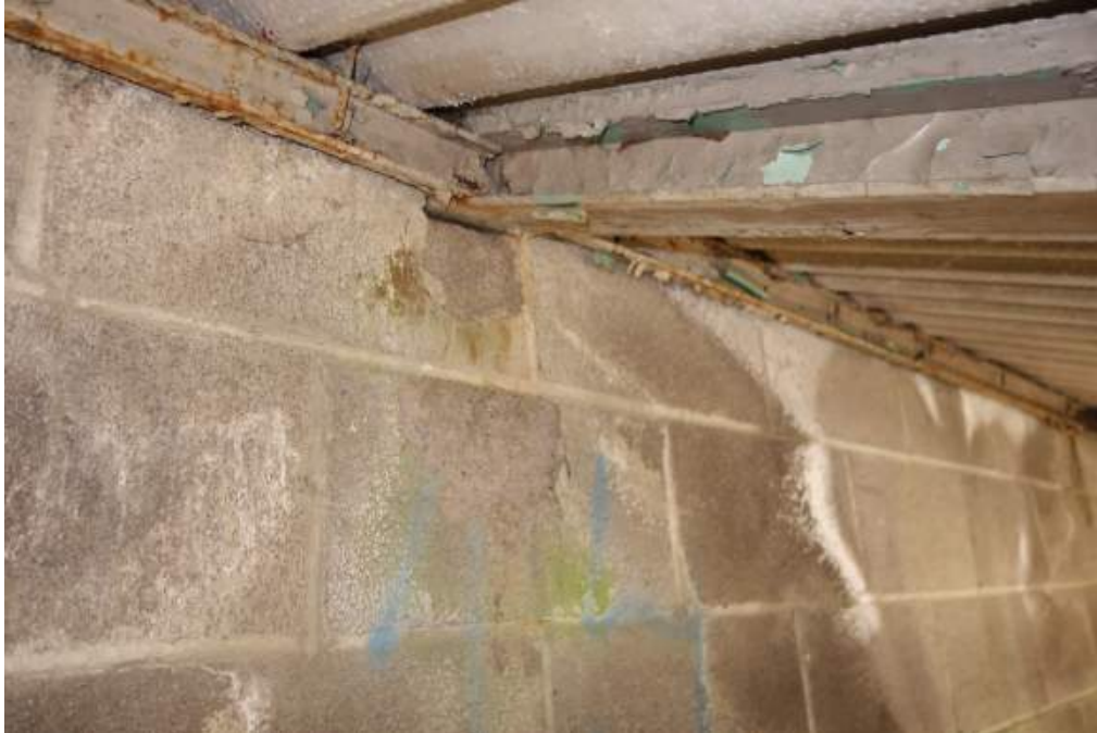
FIGURE S4U: SIGNIFICANT STEEL CORROSION AROUND AND IN MECHANICAL ROOM
