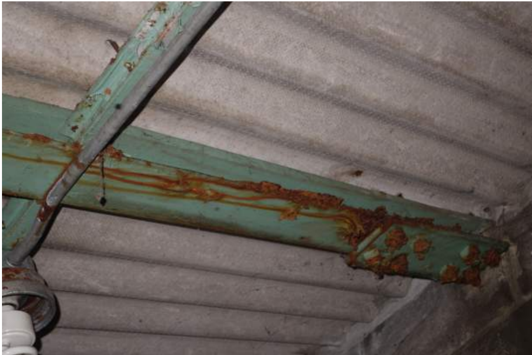
FIGURE S4L: SIGNIFICANT STEEL CORROSION AROUND AND IN MECHANICAL ROOM
