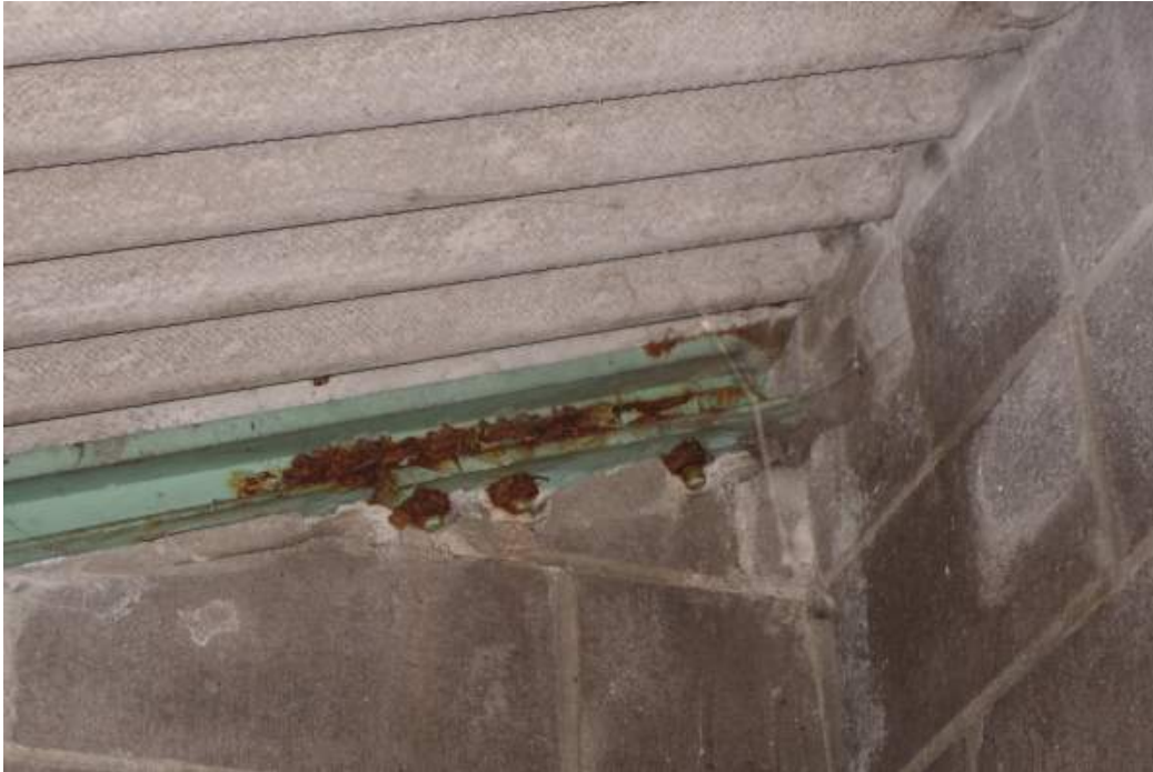
FIGURE S4M: SIGNIFICANT STEEL CORROSION AROUND AND IN MECHANICAL ROOM
