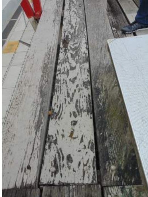
FIGURE B2D: DAMAGED / WEATHERED BLEACHER BOARDS
