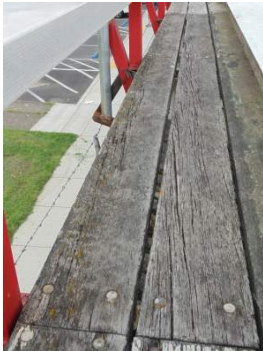
FIGURE B2C: DAMAGED / WEATHERED BLEACHER BOARDS
