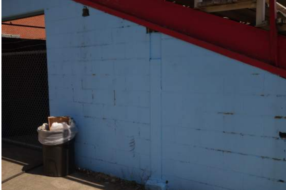
FIGURE F1C: DETERIORATION OF CMU
