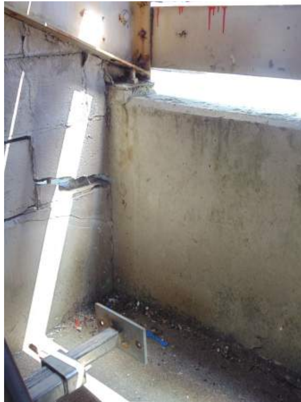
FIGURE F1D: DETERIORATION OF CMU
