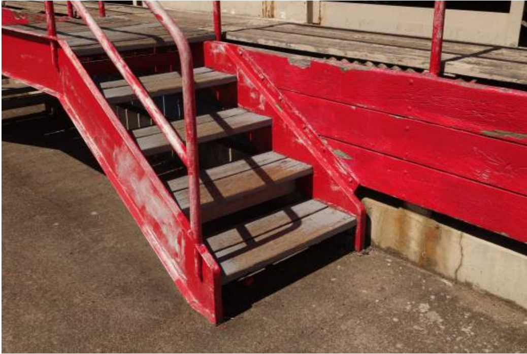
FIGURE F3B: MINOR CRACKING IN FRONT BEARING CONCRETE STEMWALL TYPICAL OF ENTIRE STEMWALL
