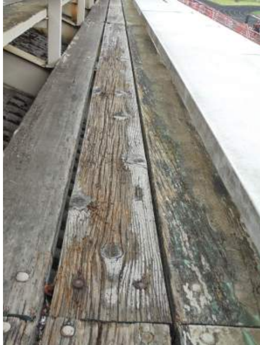
FIGURE B2B: DAMAGED / WEATHERED BLEACHER BOARDS
