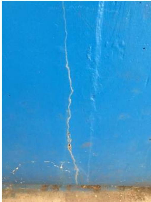
FIGURE F7A: SPALLING ALONG WITH CRACK
