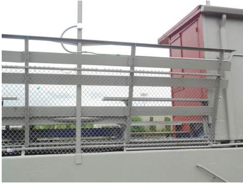
FIGURE R2: INSUFFICIENT RAILNG SPLICE
