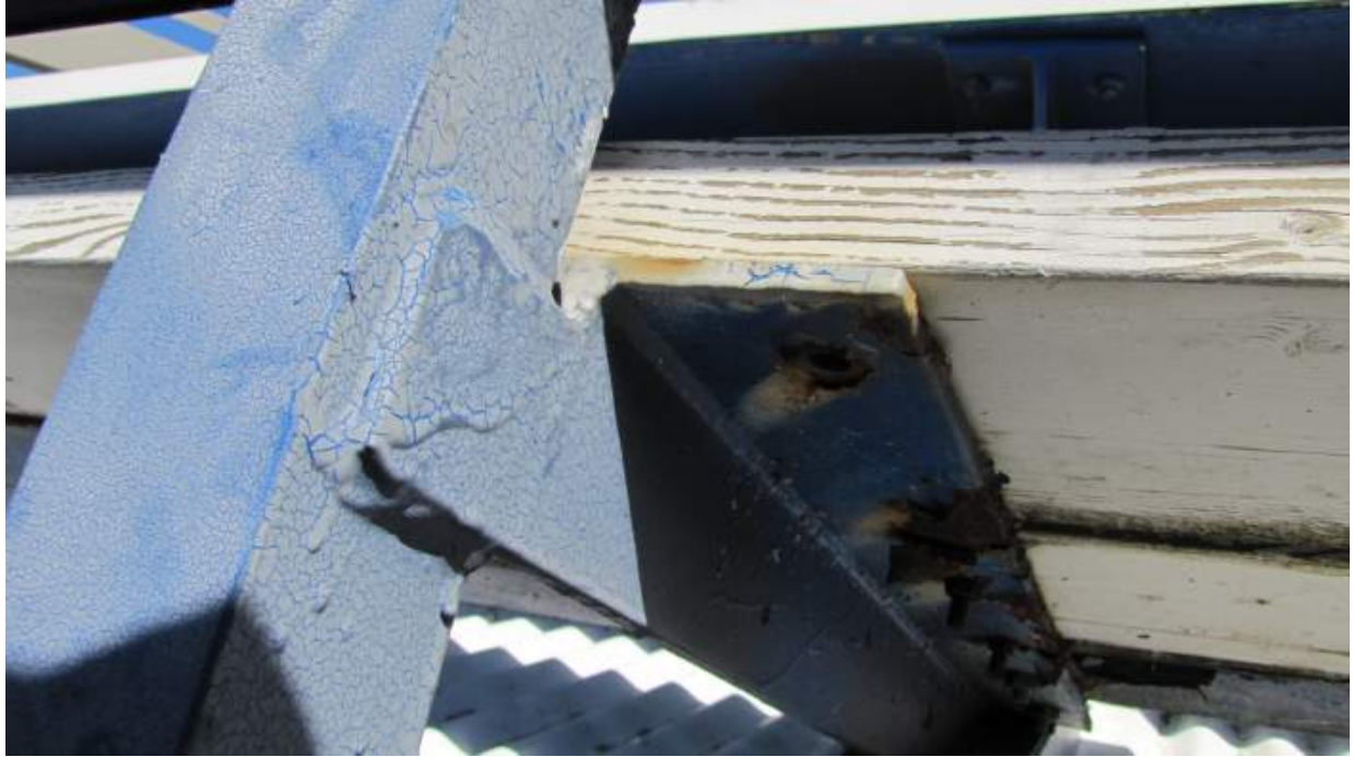
FIGURE S6: CONNECTION (BOLT AND PLATE) RUST AT BLEACHER BOARD CONNECTIONS
