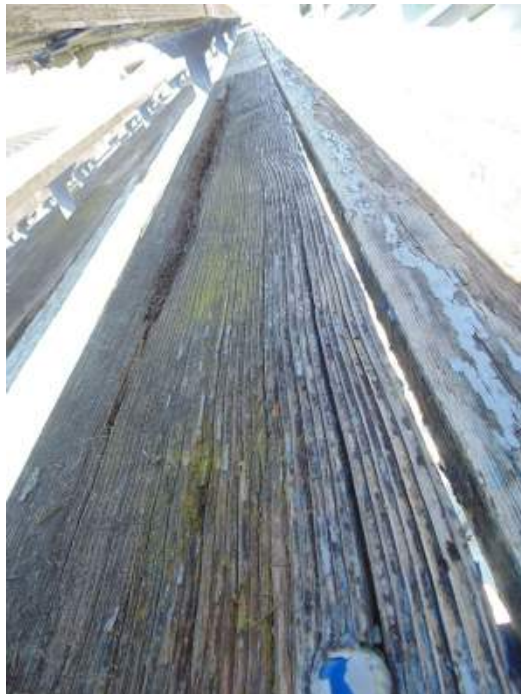
FIGURE B1B: SIGNIFICANTLY DAMAGED BLEACHER BOARDS
