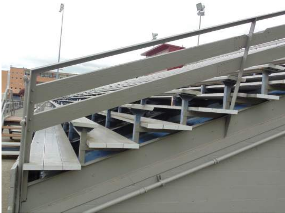
FIGURE R3C: INSUFFICIENT RAILNG SPLICE
