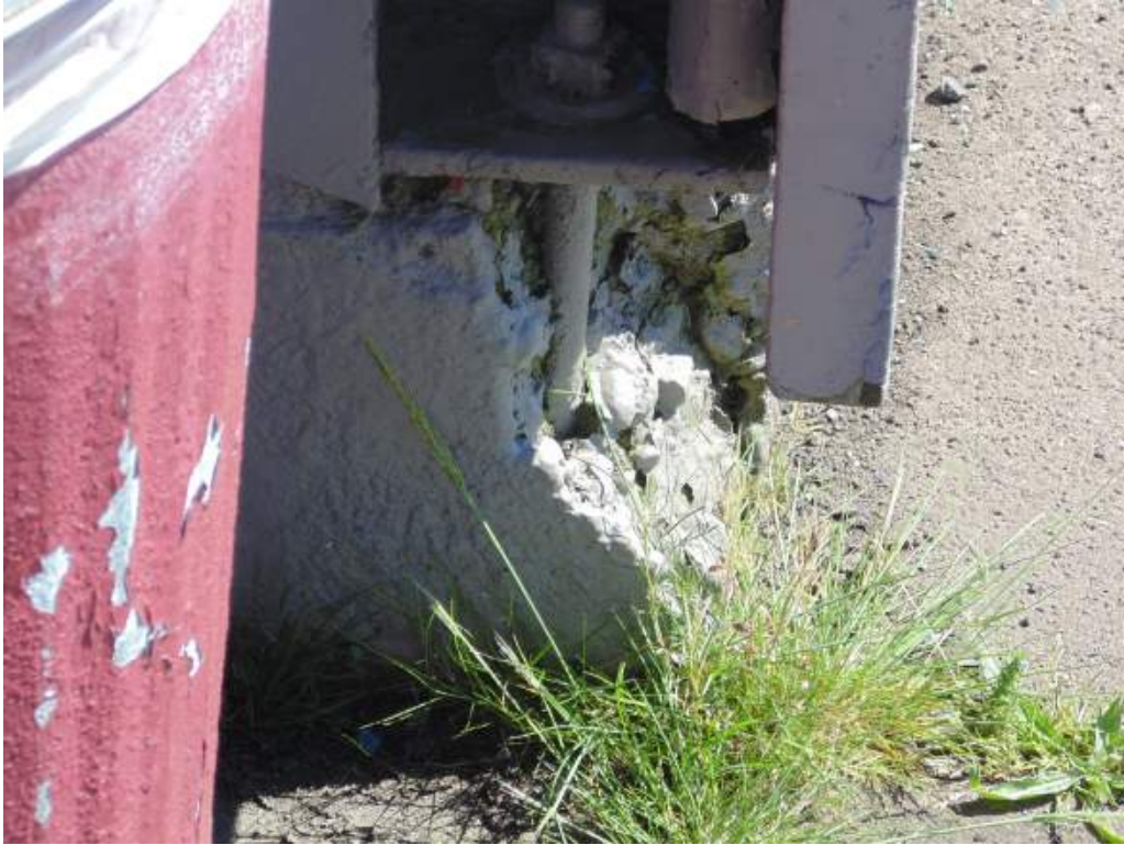
FIGURE F1A: CONCRETE STEMWALL SPALLING AT NORTH CORNER
