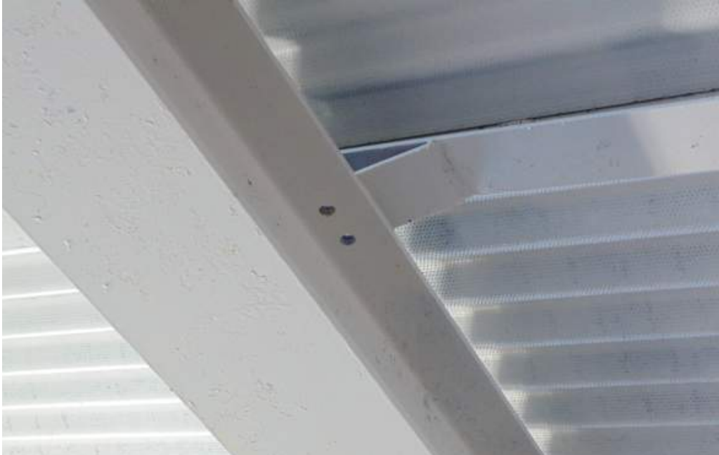
FIGURE S4: MISSING BOLTS AT STEEL RAKER TO STEEL BEAM
