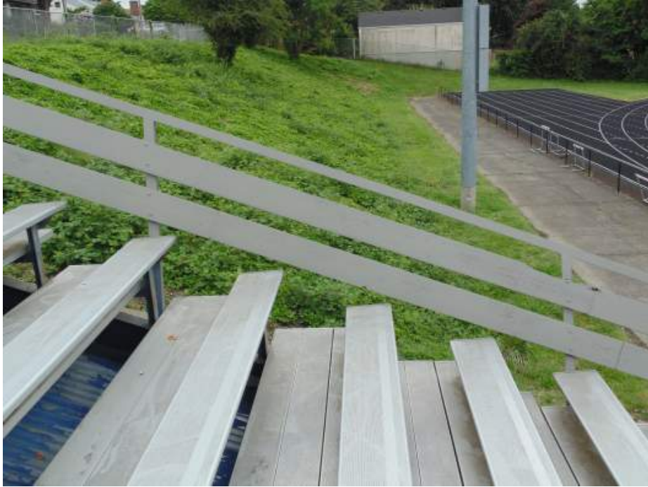
FIGURE R4: DAMAGED RAILING
