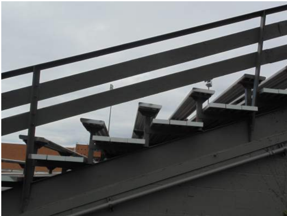
FIGURE R5A: LARGE SPACE BETWEEN RAILING AND BLEACHERS
