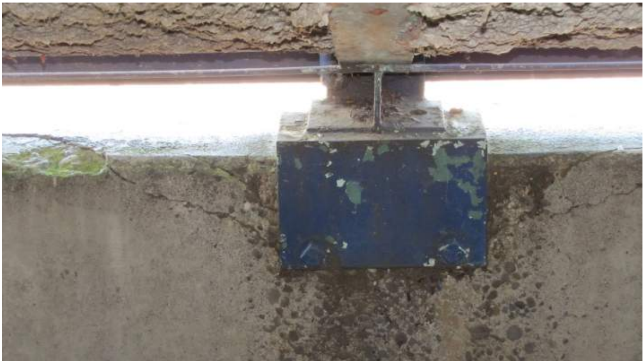
FIGURE S1B: SPALLING/CRACKING AT CONCRETE STEMWALL SUPPORTING STEEL RAKER
