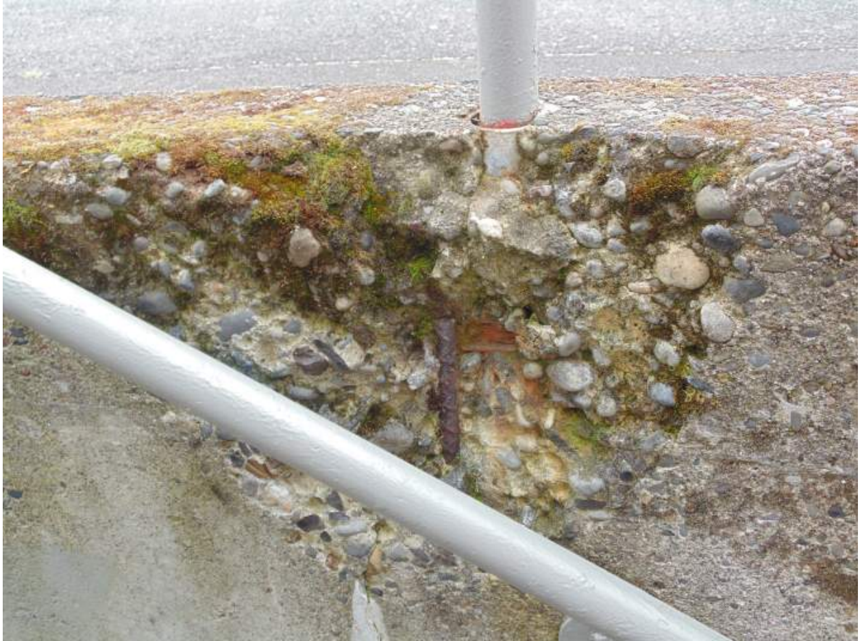
FIGURE F4: SPALLING AT EAST SIDE
