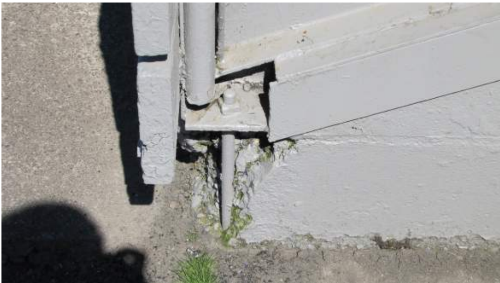
FIGURE F1B: CONCRETE STEMWALL SPALLING AT SOUTH CORNER
