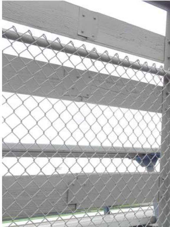
FIGURE R3A: INSUFFICIENT RAILNG SPLICE
