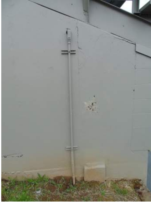
FIGURE F2: SMALL CONCRETE CRACK AT NORTH WALL PILASTER
