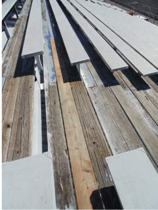
FIGURE B1C: SIGNIFICANTLY DAMAGED BLEACHER BOARDS AT FRONT OF AISLE
