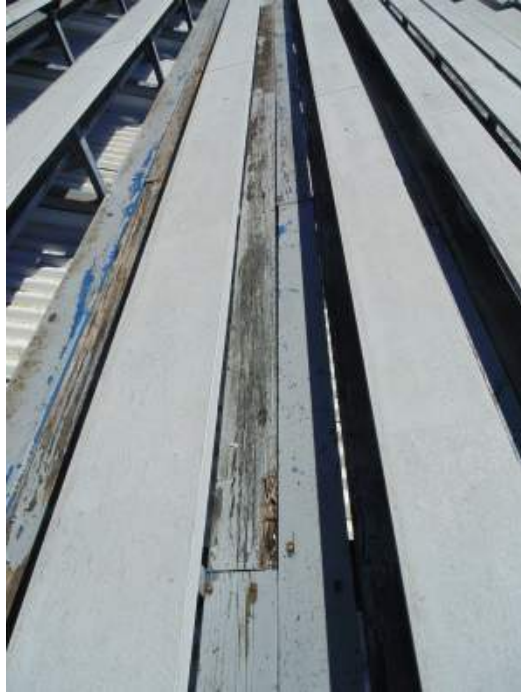
FIGURE B2B: DAMAGED/WEATHERED BLEACHER BOARDS
