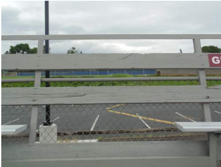
FIGURE R1B: DAMAGED RAILING
