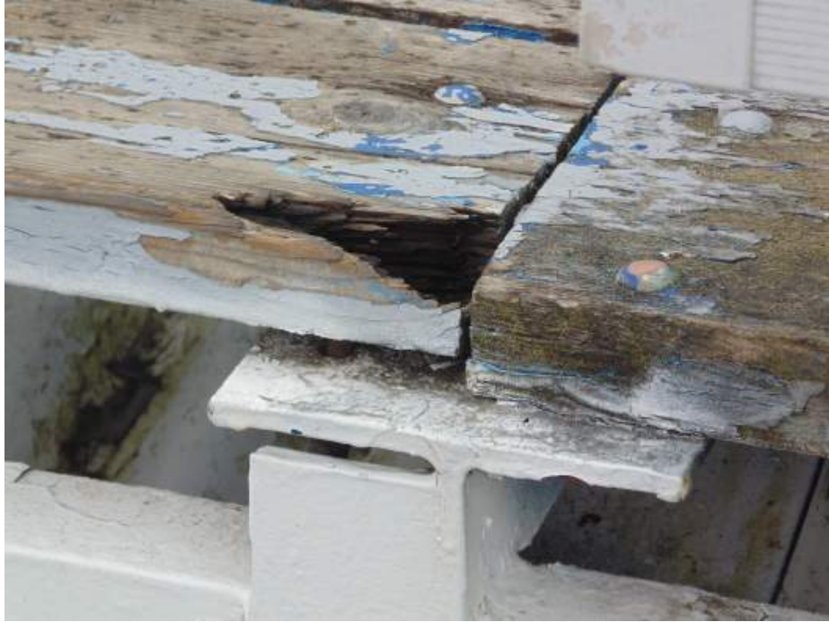
FIGURE B6B: SIGNIFICANT BLEACHER BOARD DAMAGE AT CONNECTION
