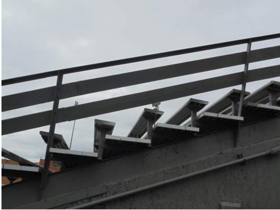
FIGURE R3B: INSUFFICIENT RAILNG SPLICE
