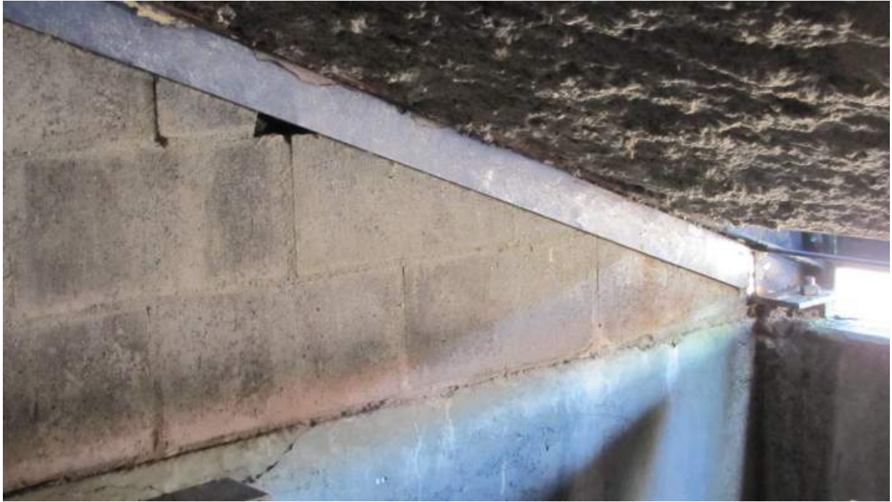
FIGURE S1A: SPALLING AT FRONT CONCRETE STEMWALL SUPPORTING STEEL RAKER
