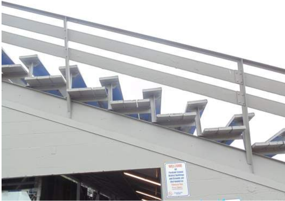
FIGURE R5B: LARGE SPACE BETWEEN RAILING AND BLEACHERS
