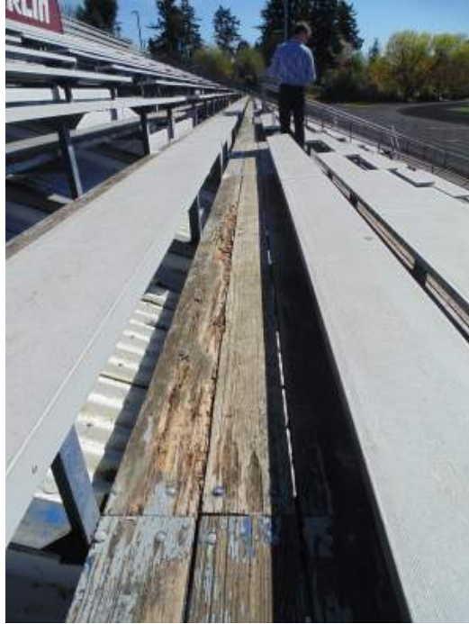
FIGURE B1A: SIGNIFICANTLY DAMAGED BLEACHER BOARDS
