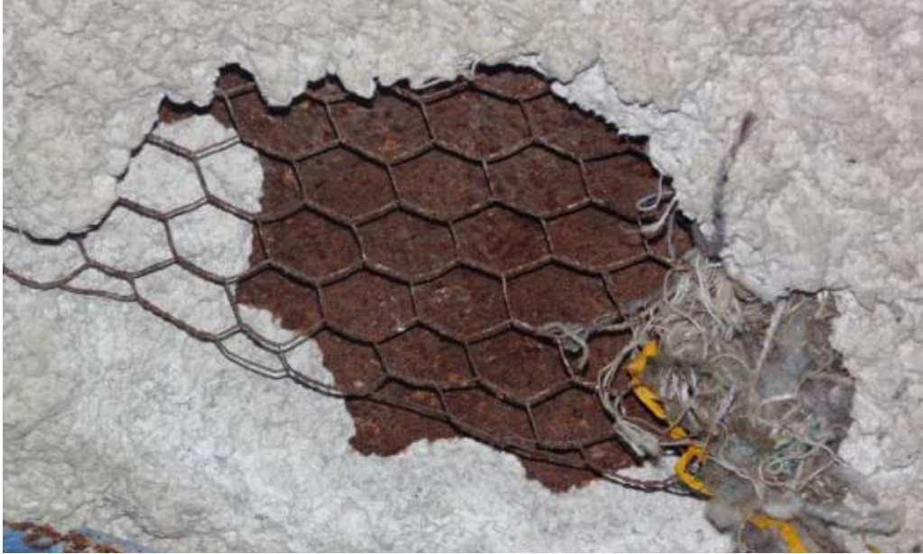
FIGURE S5C: POTENTIAL STEEL BEAM RUST DUE TO WATER INTRUSION
