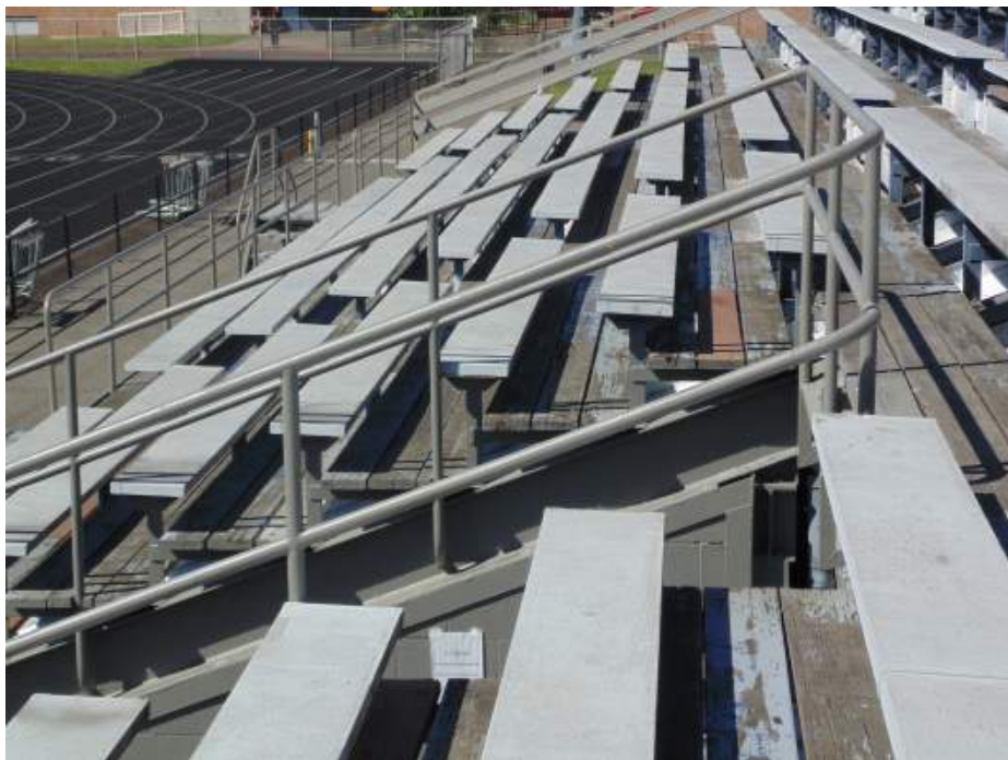
FIGURE R5C: LARGE SPACE BETWEEN RAILING AND BLEACHERS
