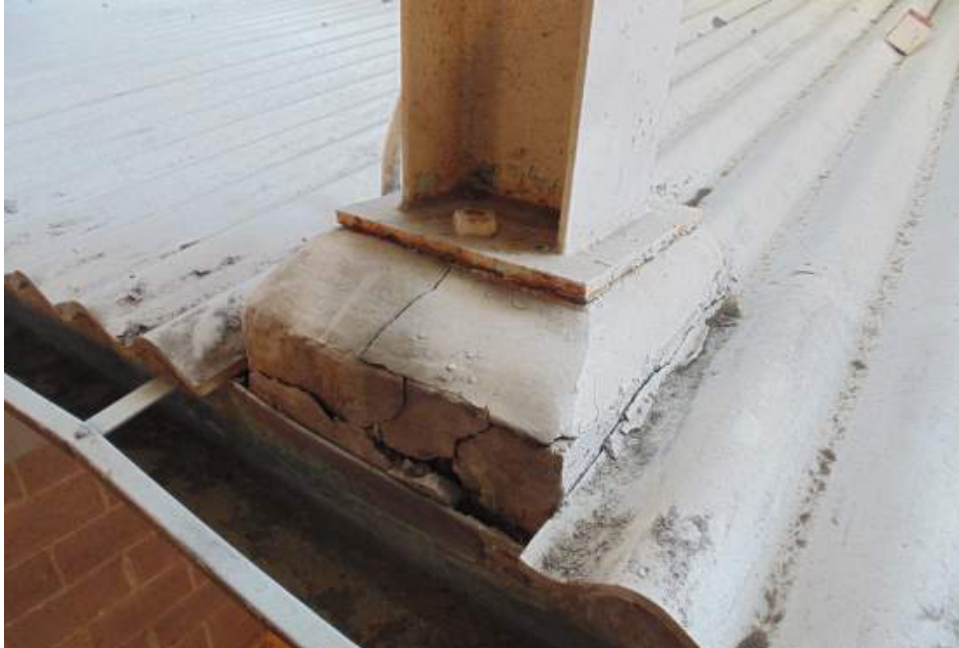
FIGURE S2: CRACKING OF GROUT AT STEEL COLUMN BASE PLATE
