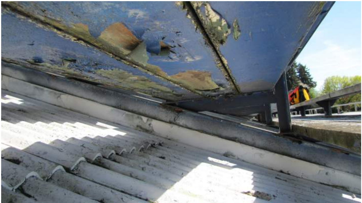
FIGURE B7: DETERIORATED PAINT AT UNDERSIDE OF BLEACHER BOARDS
