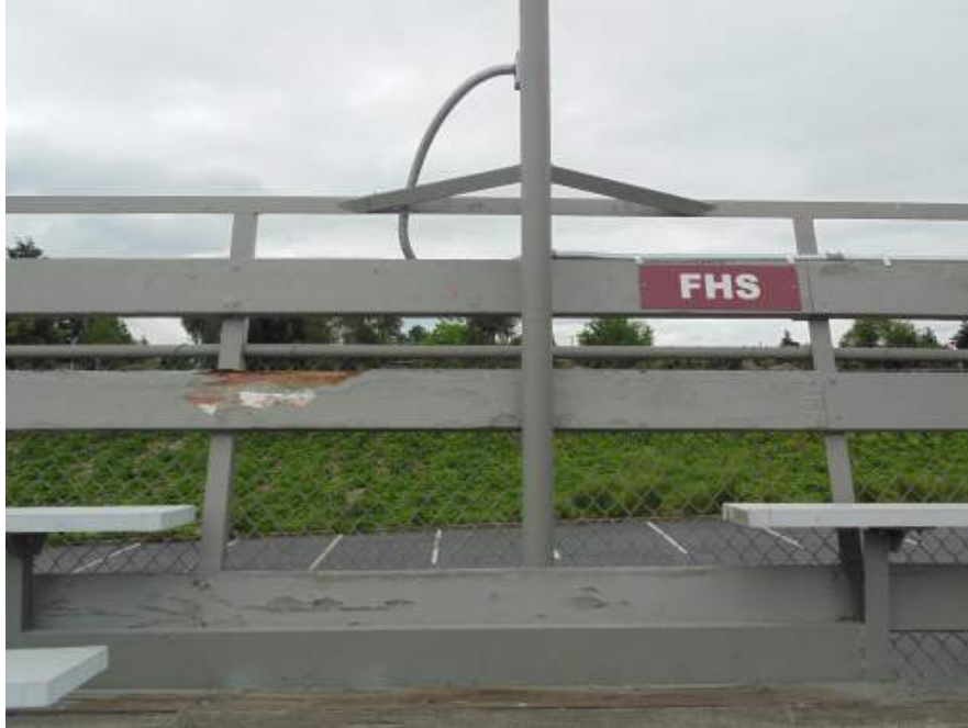
FIGURE R1A: DAMAGED RAILING
