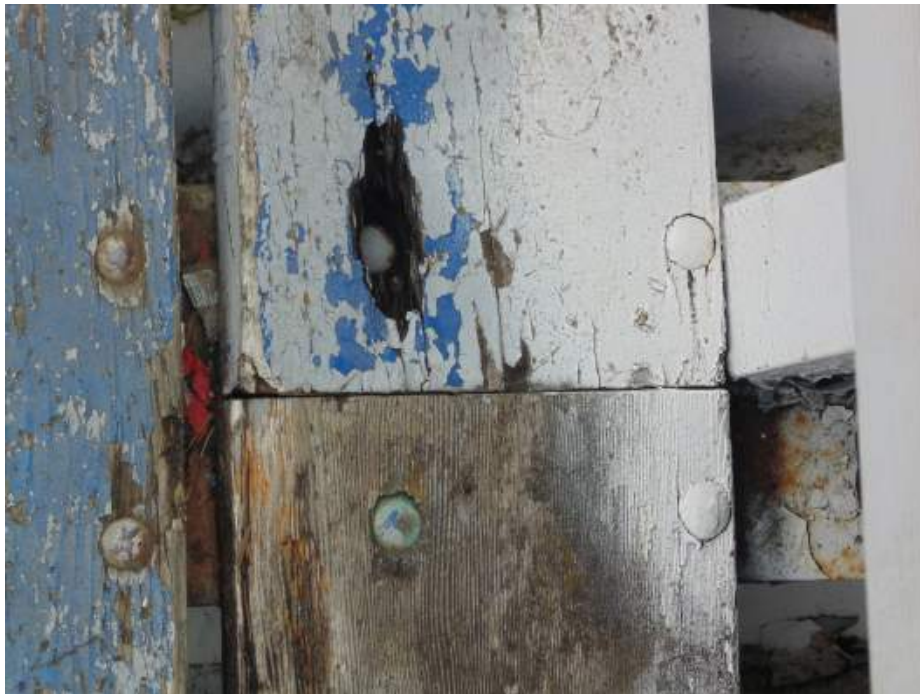
FIGURE B6A: SIGNIFICANT BLEACHER BOARD DAMAGE AT CONNECTION
