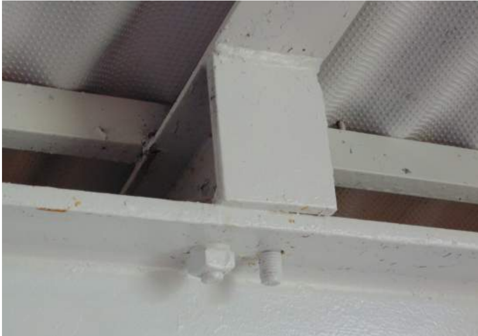
FIGURE S3: MISSING NUT AT STEEL RAKER TO STEEL BEAM
