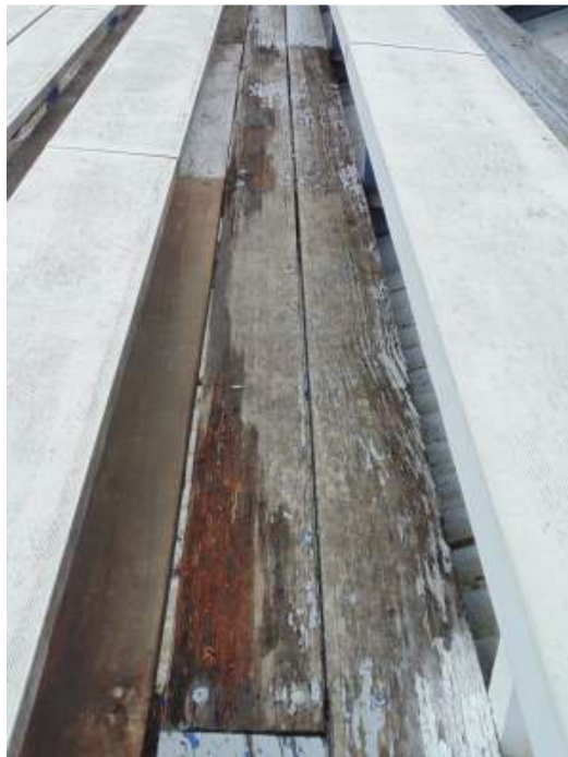
FIGURE B2A: DAMAGED/WEATHERED BLEACHER BOARDS
