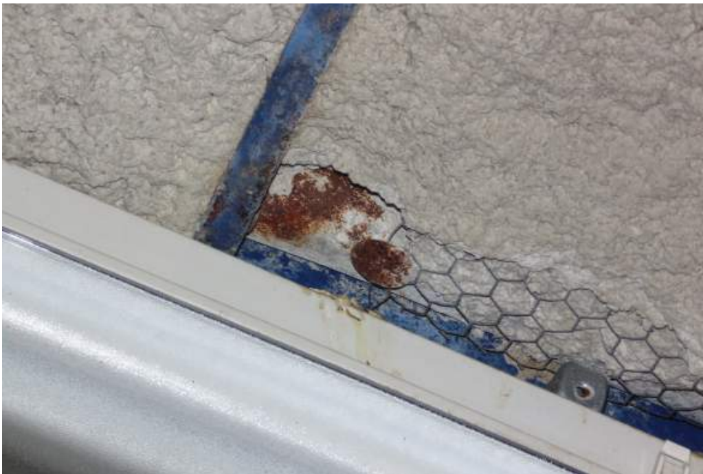
FIGURE S5A: POTENTIAL STEEL BEAM RUST DUE TO WATER INTRUSION
